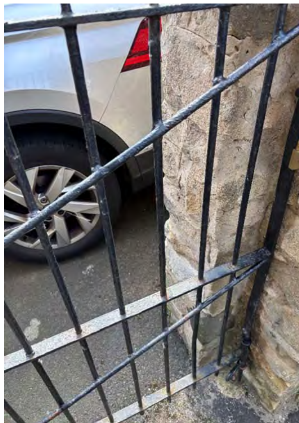
Evidence of flaking paint and rusting to gate.
