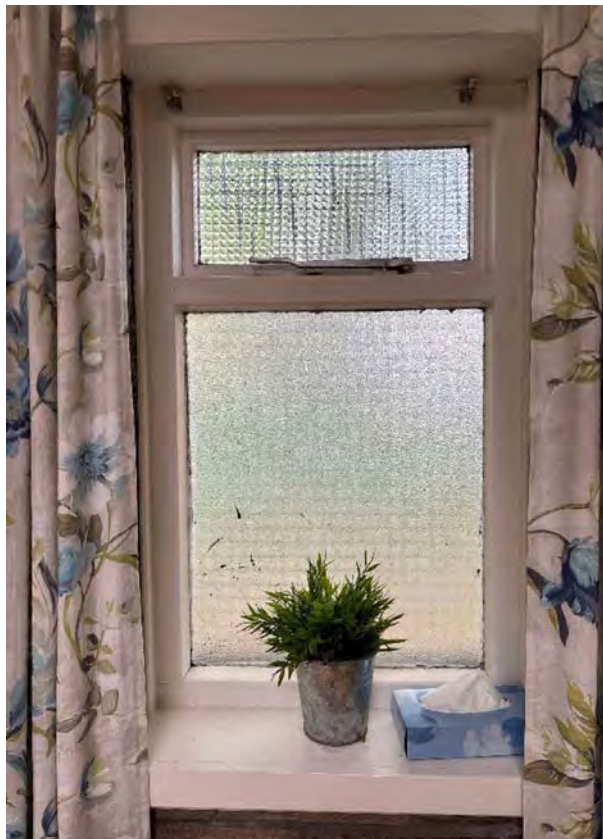
Dirt / paint markings to frames.
