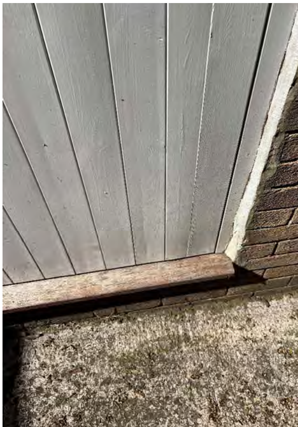
Flaking paint to door threshold
