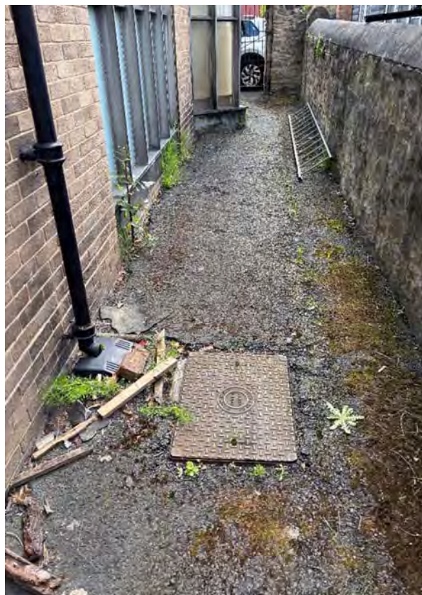
Rubbish and debris to be cleaned from rear churchyard/garden.
