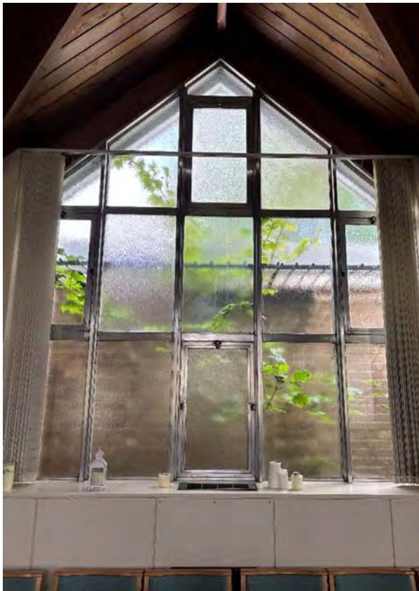
Vegetation growth visible to void in centre of church. Refer to Roof Coverings for info.
