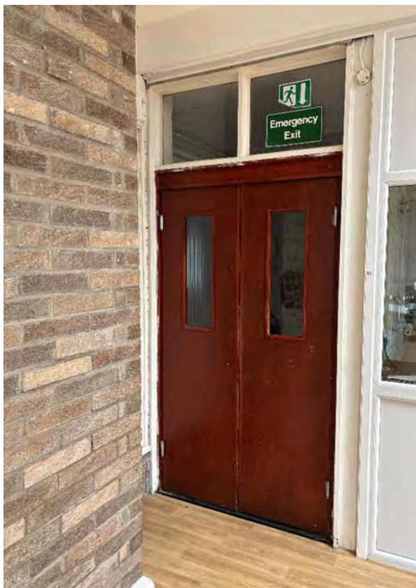
Clearance of double doors inadequate for fire escape doors.
