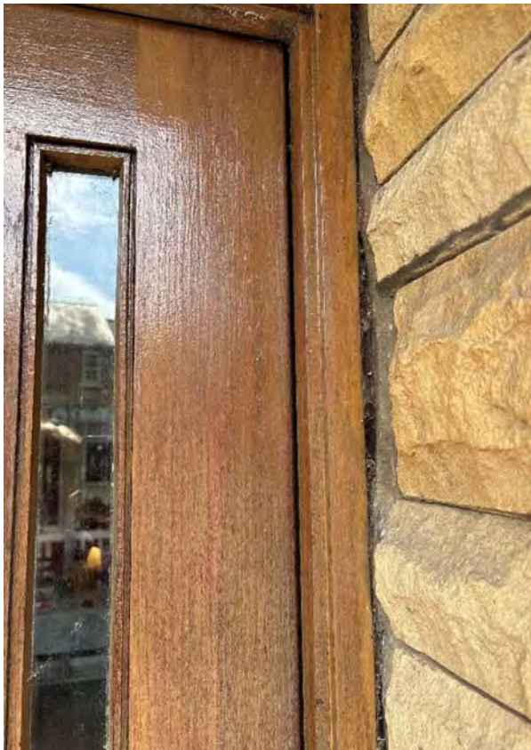
Loss of seal around door edge
