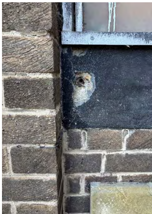
Evidence of spalling to concrete lintel.
