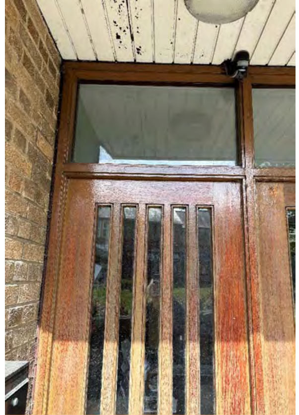
Loss of finish to doors
