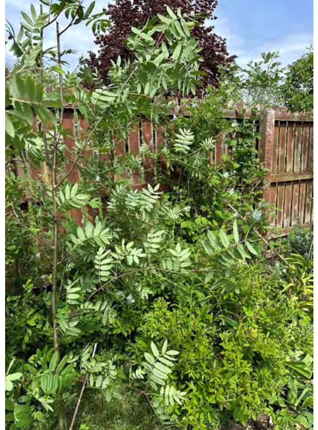
Overgrowth of vegetation to rear boundary
