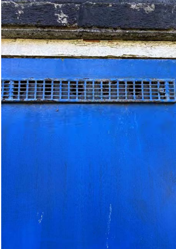
Rusting to grilles
