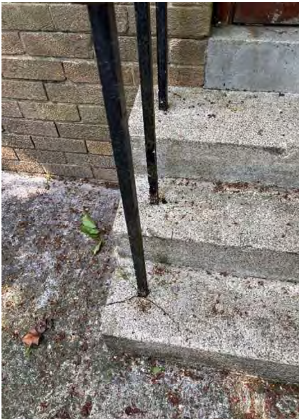
Evidence of cracking around handrail fixing.
