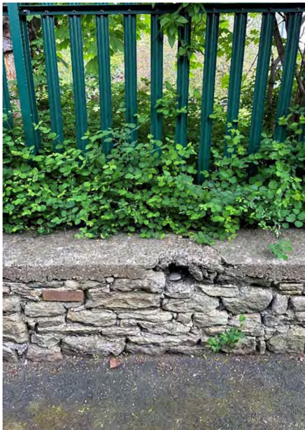
Example of loss of stone from iron fixing (occurs across whole wall)
