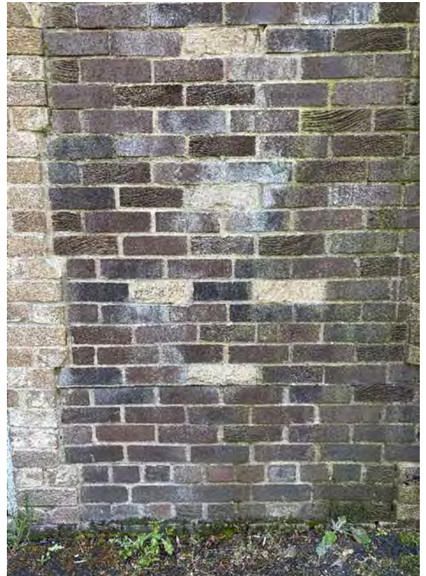
Efflorescence visible on this section of the elevation.
