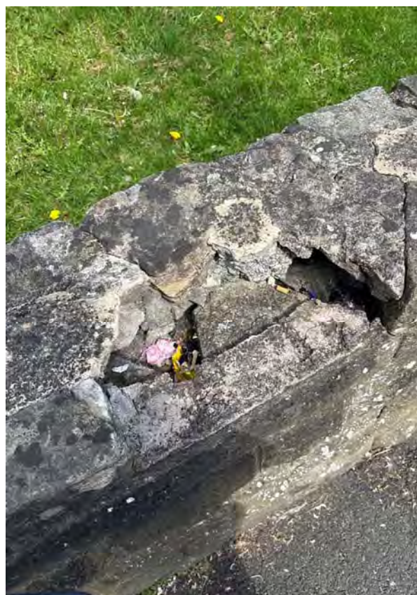
Close view of missing stone area.
