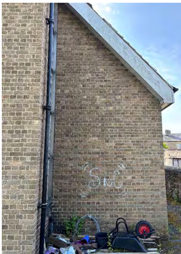
Overview of right area of elevation with graffiti shown to centre.
