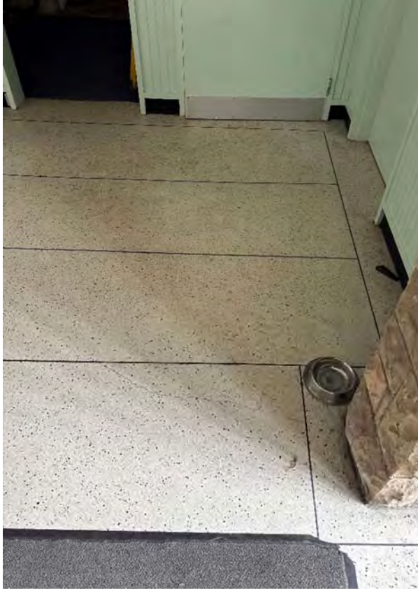
Hairline cracking continues beyond entrance doors
