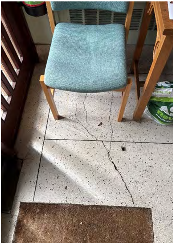
Cracking to right side of door.
