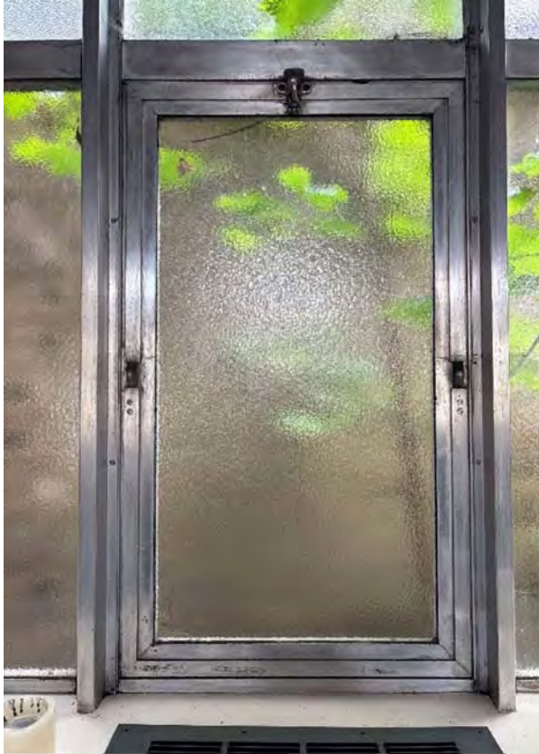
Example deterioration to frames
