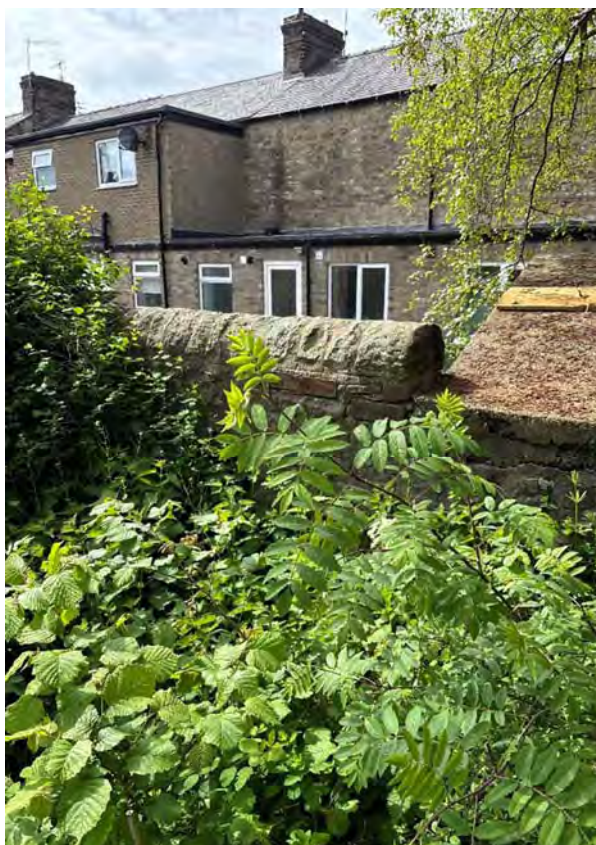
Areas of stone boundary not accessible due to vegetation overgrowth
