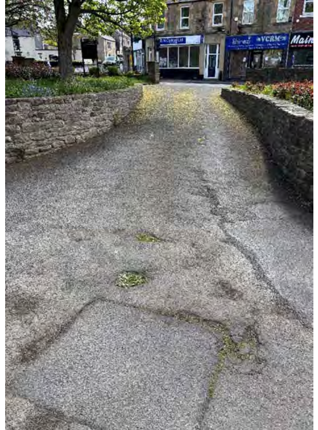
Potholes and vegetation growth to tarmac.
