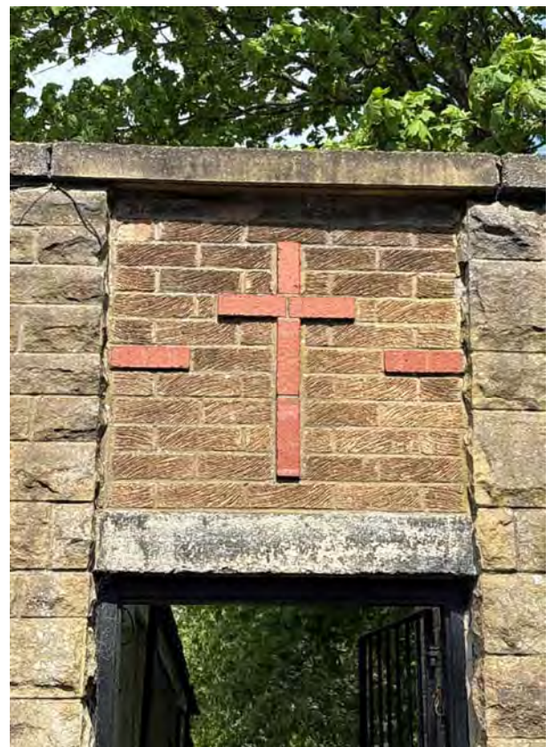
Loss of pointing to coping stones and between stone and brick connection.
