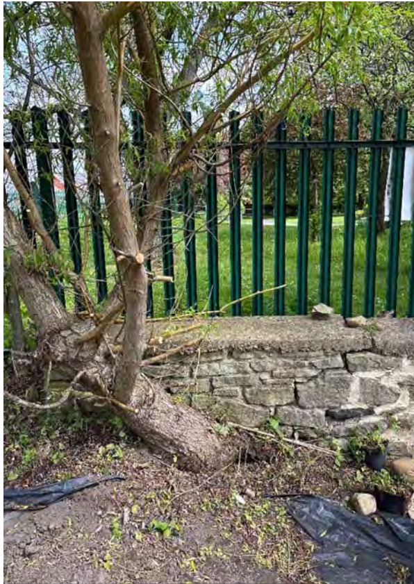
Tree roots impacting on stone boundary wall.
