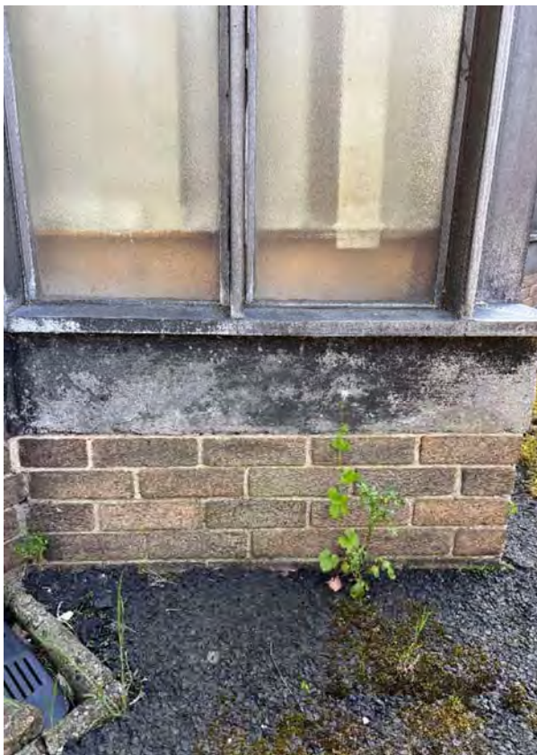
Deterioration of concrete cill
