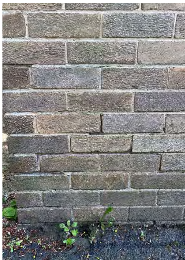
Area of loss of pointing to lower left wall
