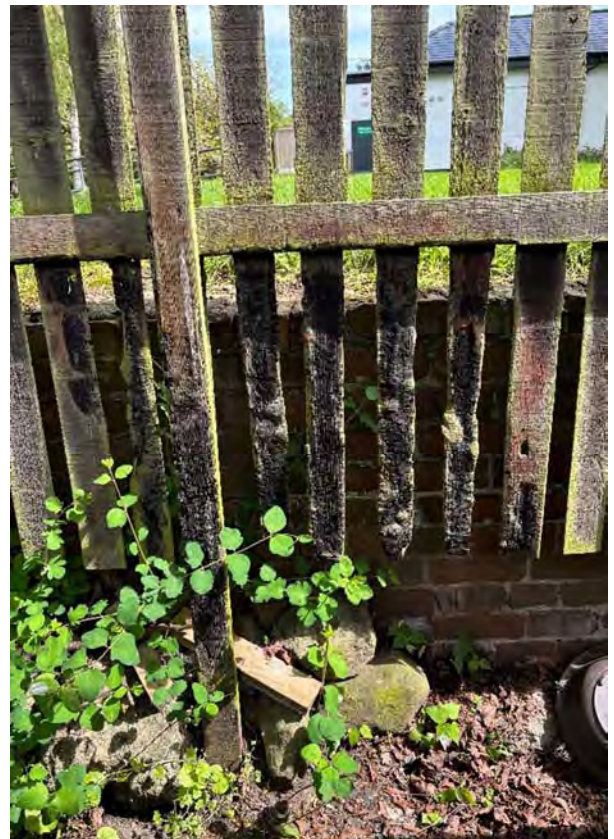
Rotten sections of timber fence.
