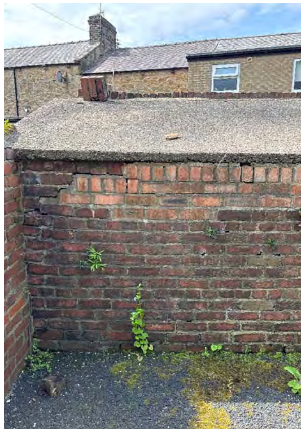
Significant cracking to brick wall
