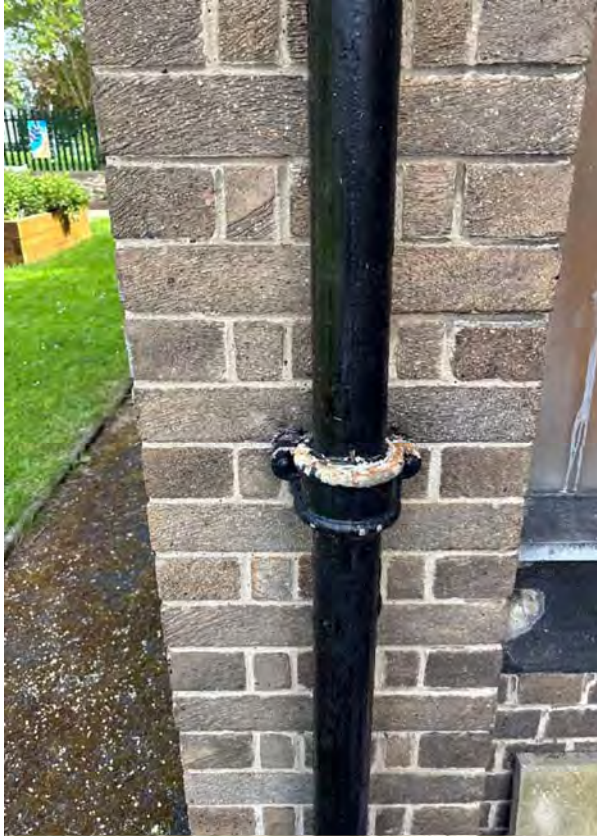
Example of flaking / rust to downpipe on West Elevation.
