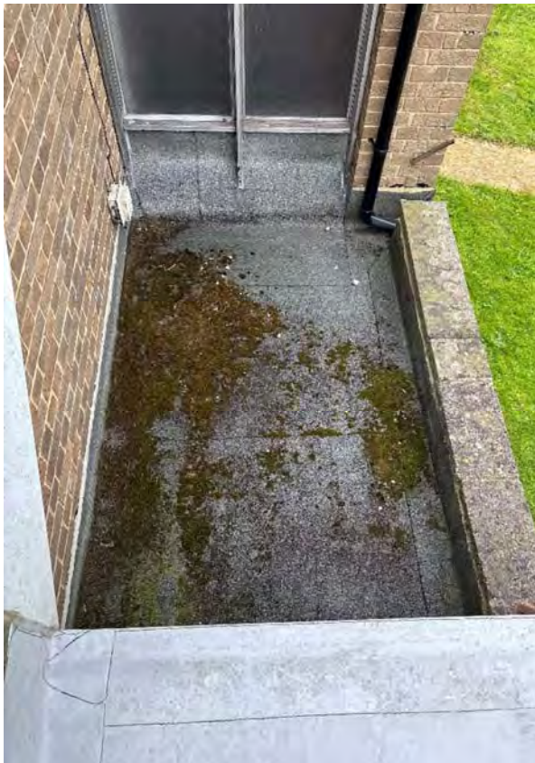
Moss growth to Boiler House Roof
