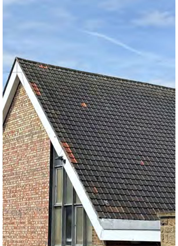
Evidence of replacement non matching slates.
