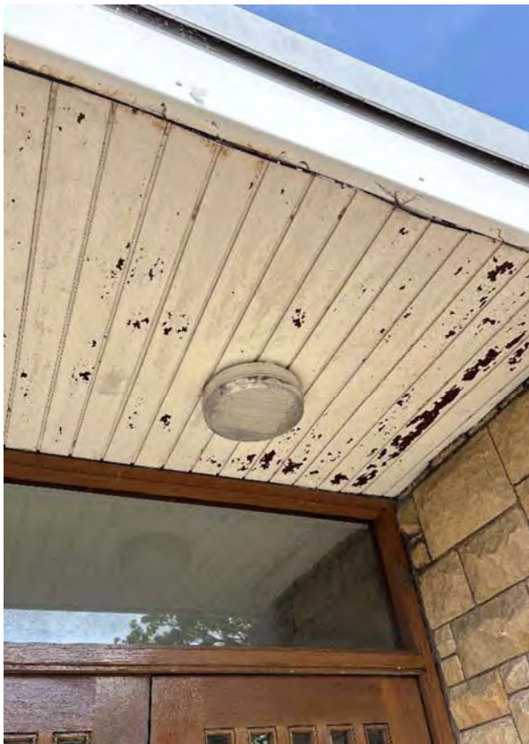
Loss of paint to ceiling area of entrance.
