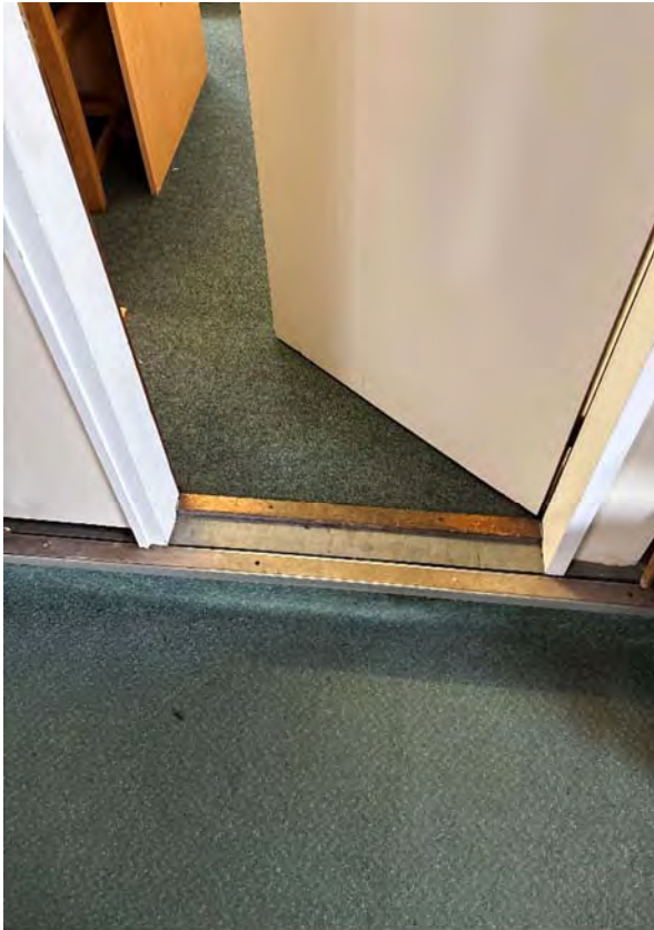
Threshold step into office. Should be clearer to prevent trips.
