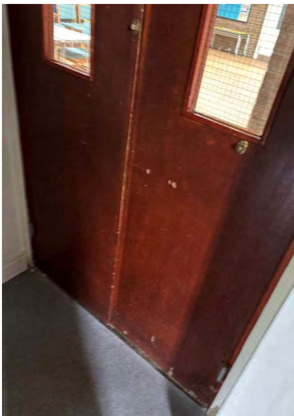
Example flaking paint / minor damage to doorset.
