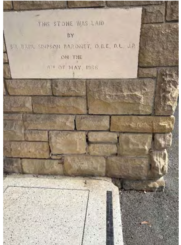
Loss of pointing to entrance area of stone wall.
