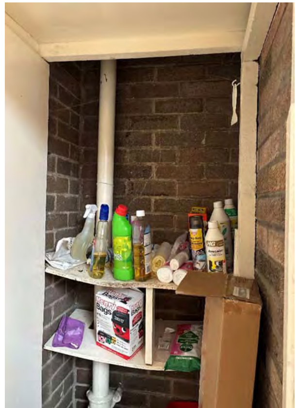
Storage cupboard shelving warping
