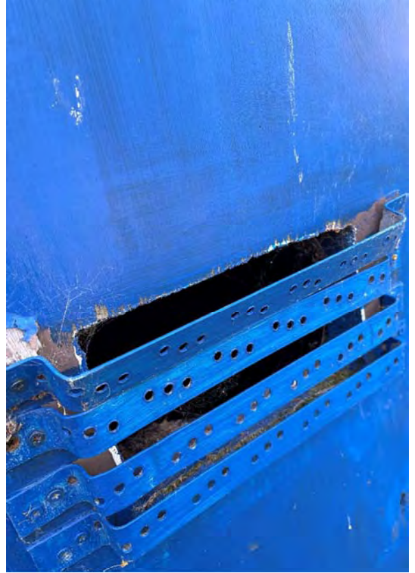
Open Vent Area
