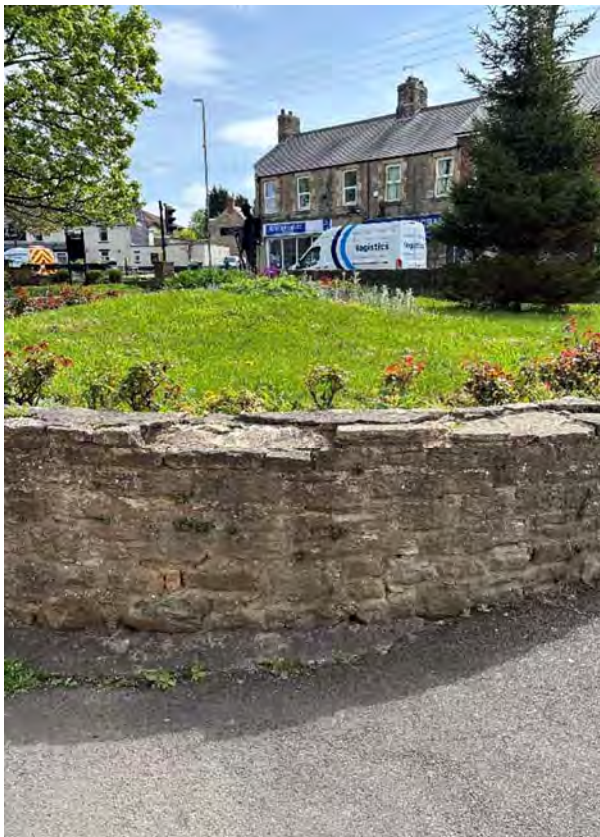
Poor condition of coping stones and upper courses.
