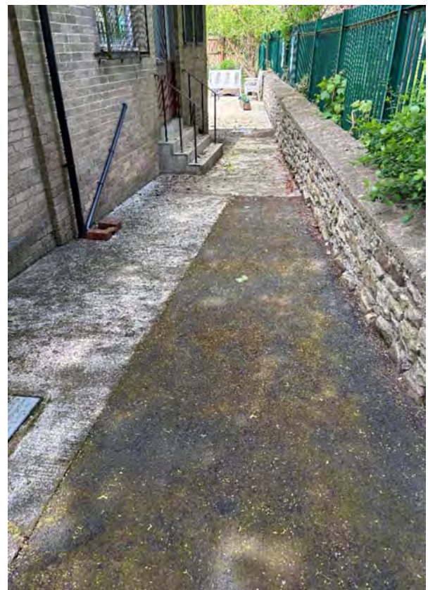
Changes to floor finish around garden creating some uneven surface finishes.
