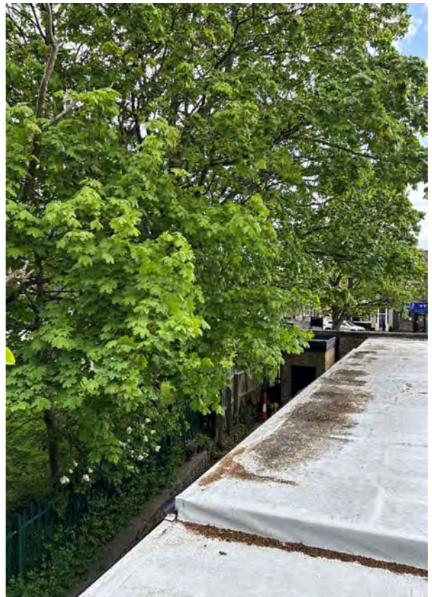
Debris and Staining to Roof from Overhanging Trees
