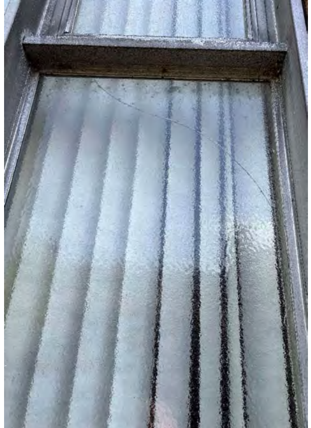
Cracked pane of glass.
