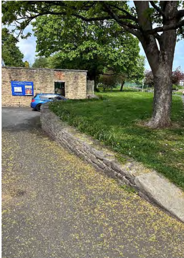
Areas of open joints to stone wall. Monitor to establish if any movements to wall.
