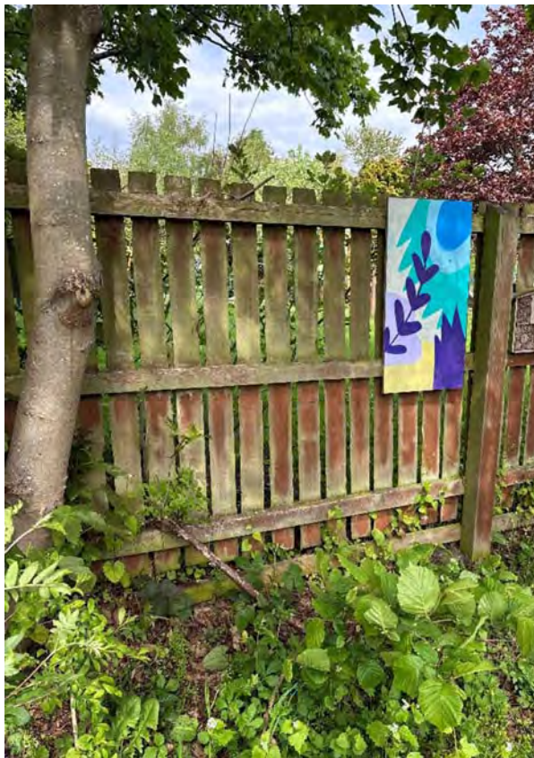
Significant weathering to fence posts and panels
