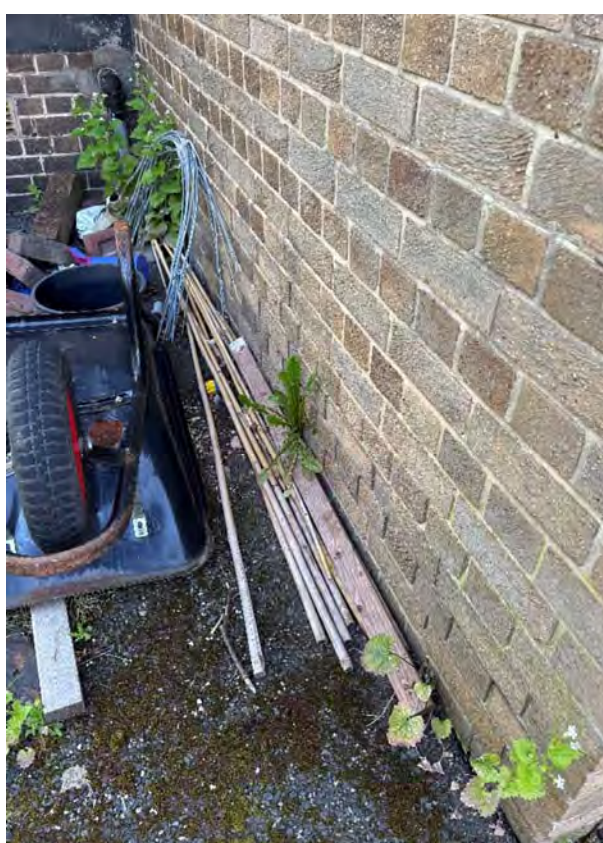
Items stored in front of elevation.
