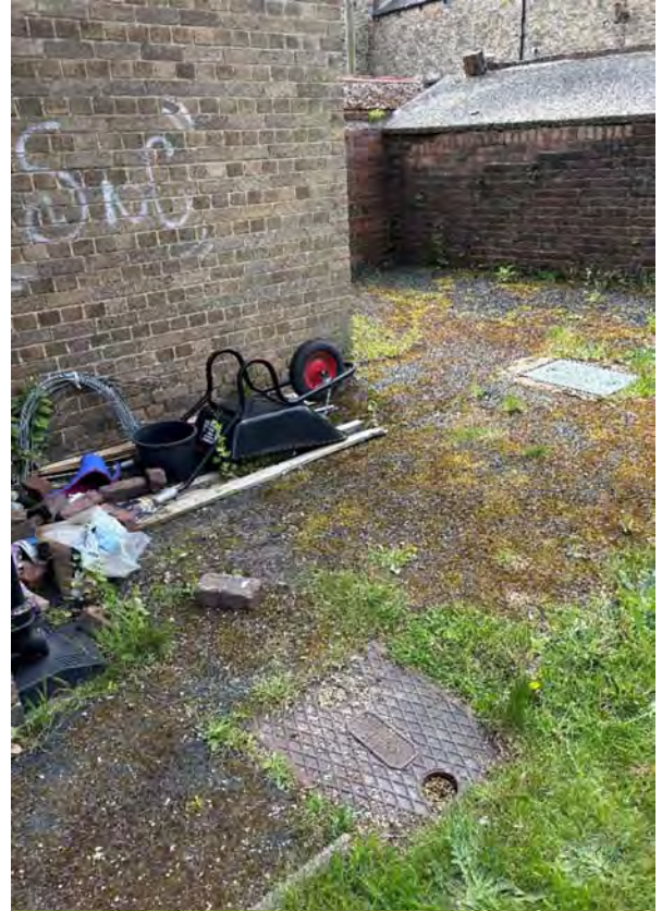
Moss / Weed growth to paved area surrounding church.
