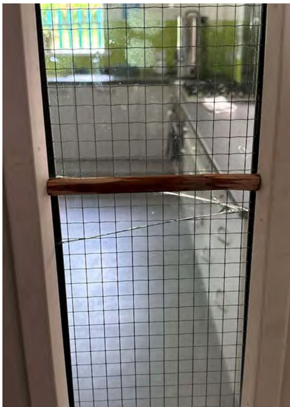
Crack to Fire Door vision panel with ad hoc repair.
