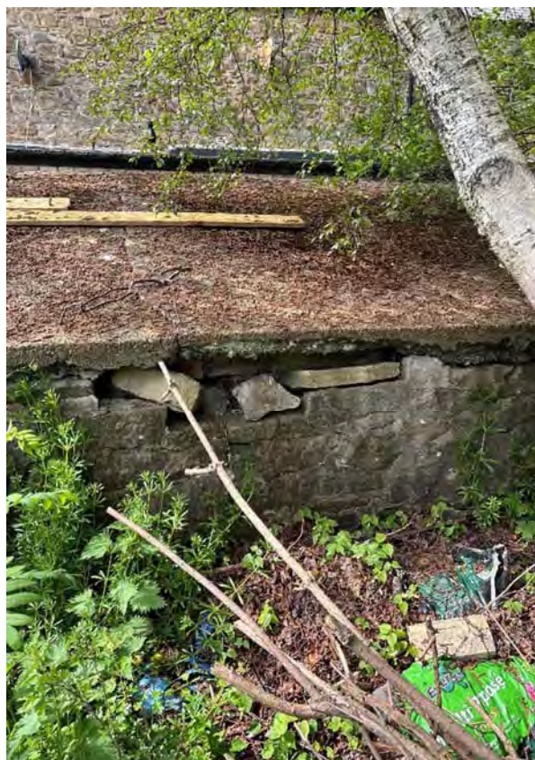
Significant deterioration to stone boundary wall.
