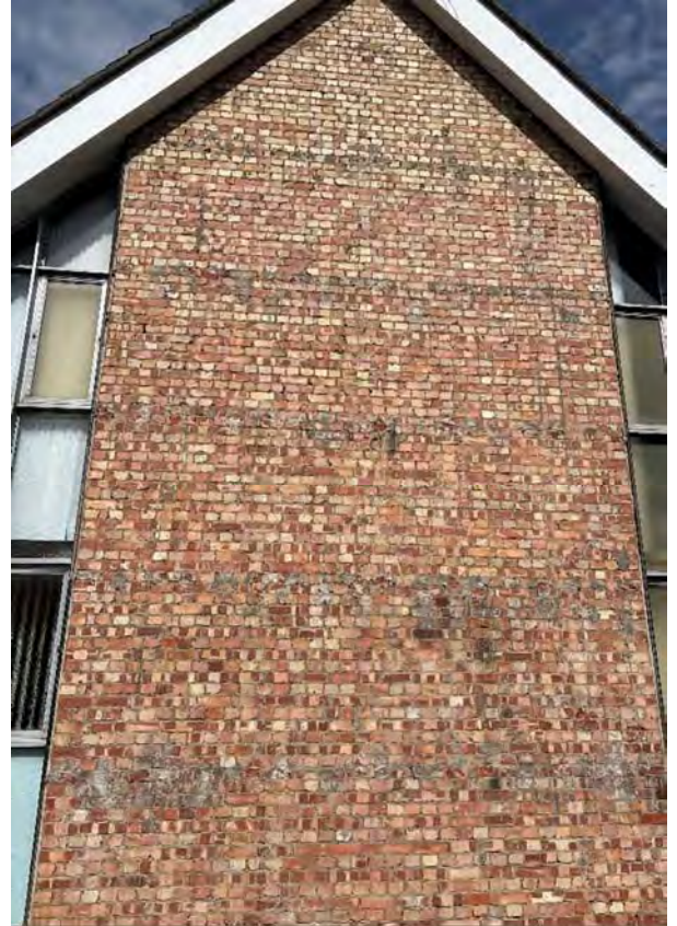
Area of exposed brickwork where slates previously were.
