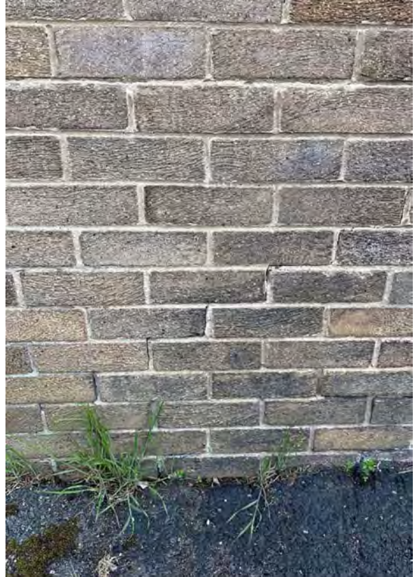
Area of stepped cracking
