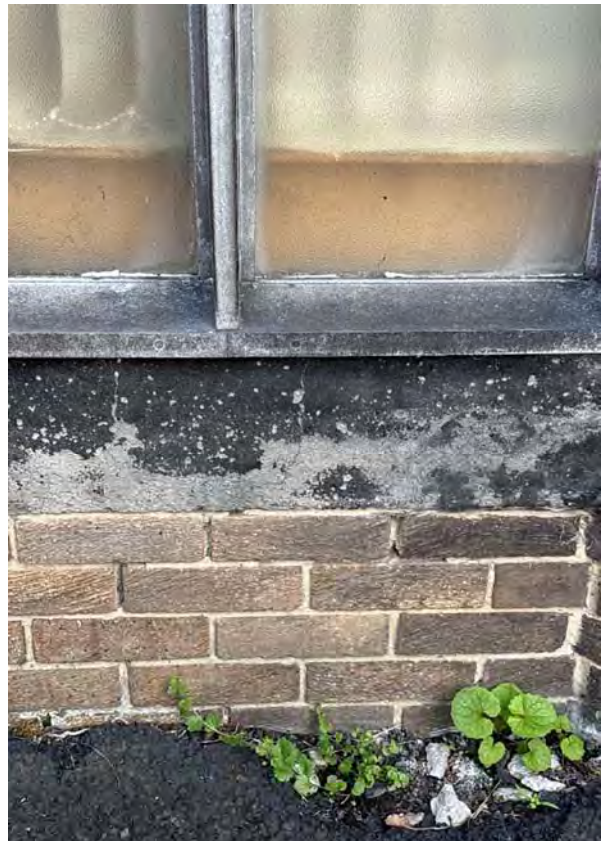
Other example area of deterioration of cill and loss of pointing.
