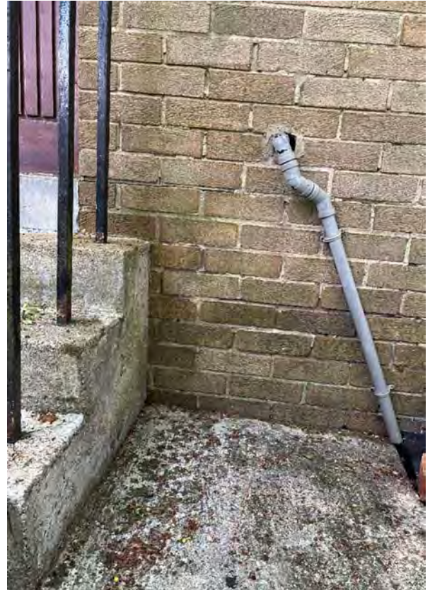
Example area where loss of pointing occurs around pipe
