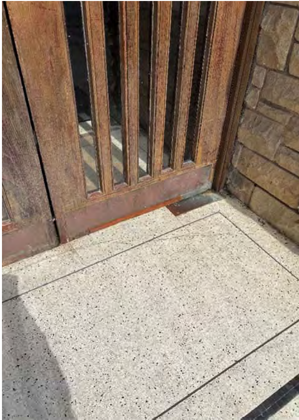
Cracking to terrazzo flooring
