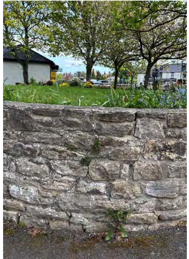
Areas of cracking and open joints visible to stone retaining walls.
