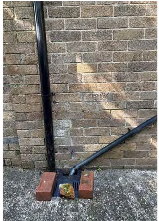
Example area of loss of pointing around pipes
