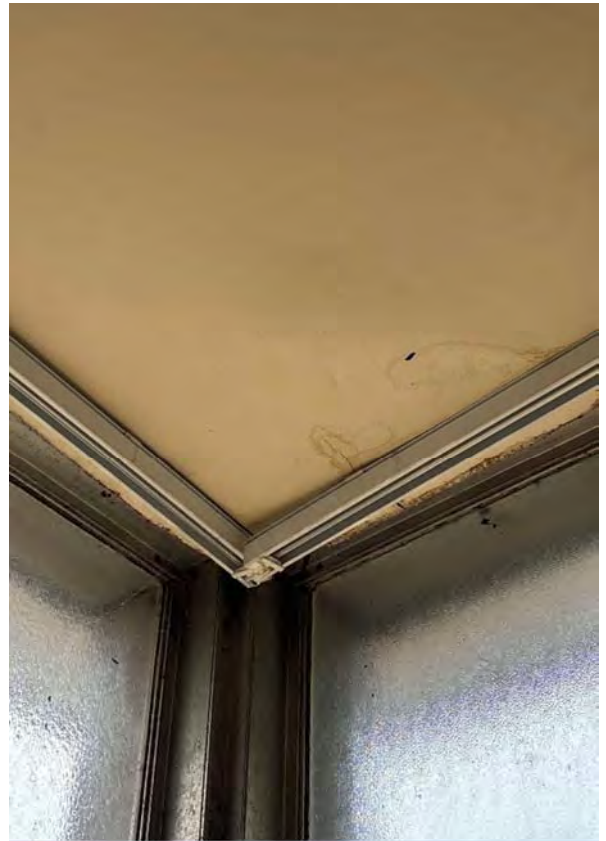
Areas of staining to ceiling of windows.
