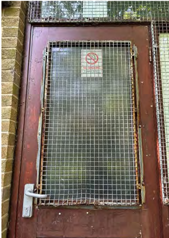
Rusting of metal security grilles
