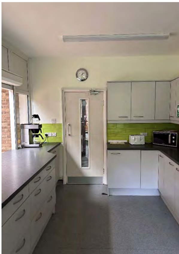
Door Stop use visible to fire door.
