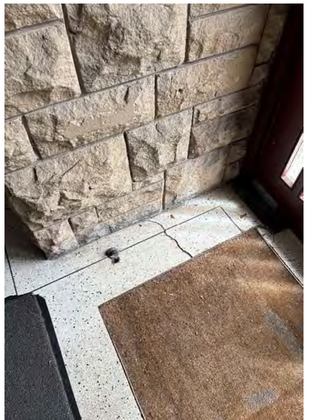
Cracking to left side of door.
