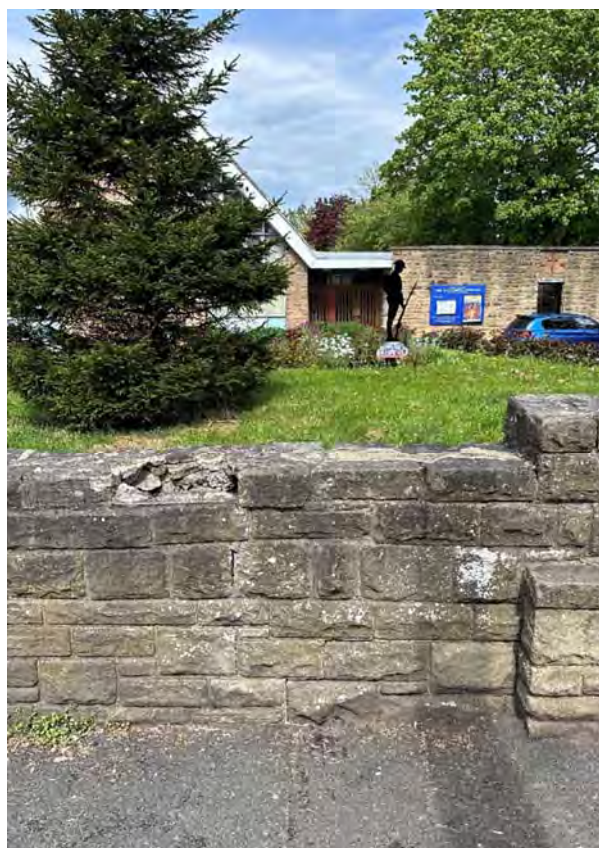
Area of missing stone to public pavement boundary wall.
