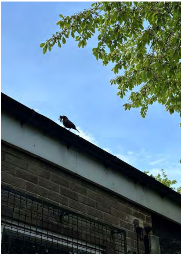
Birds gathering nesting materials from gutters – require clearing.
