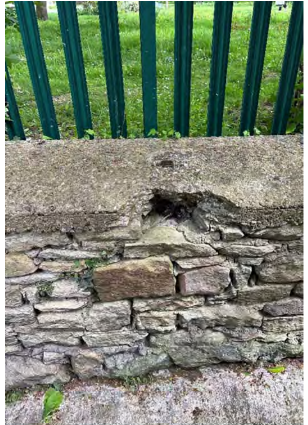
Example of loss of stone from iron fixing (occurs across whole wall)
