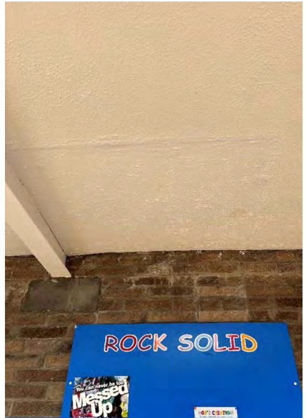
Example of uneven finishes to textured ceiling surface.
