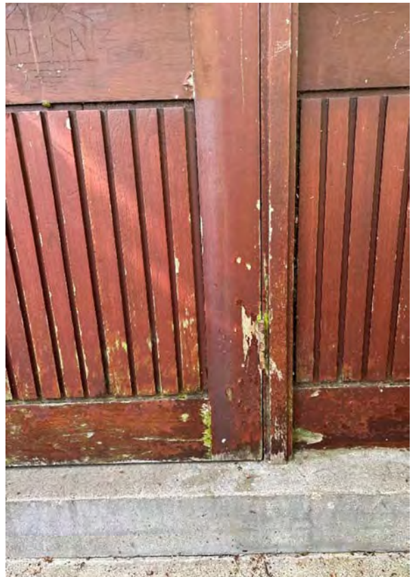
Area of flaking paint to doors
