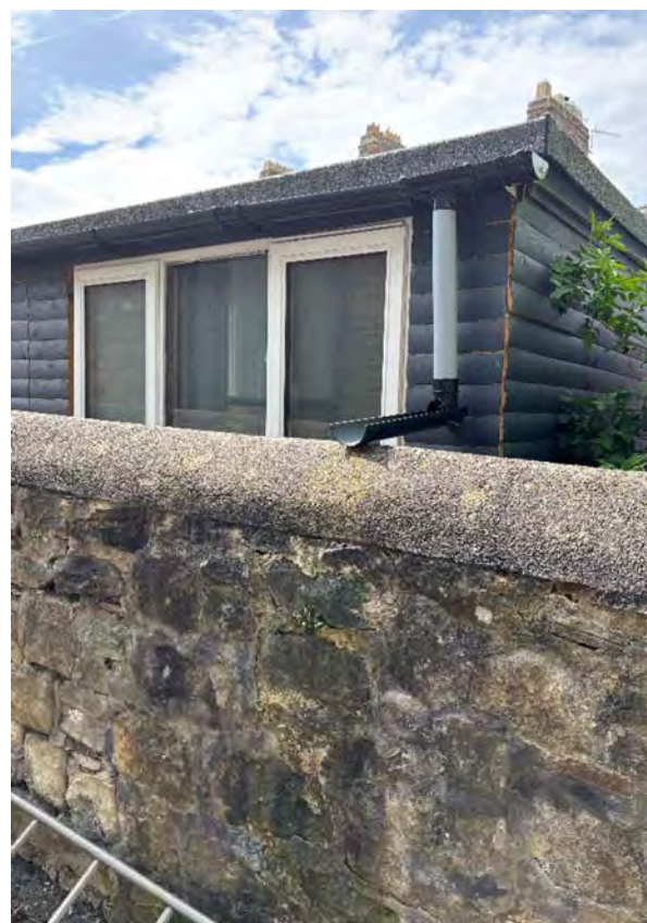
Neighbour draining rainwater over stone boundary wall.
