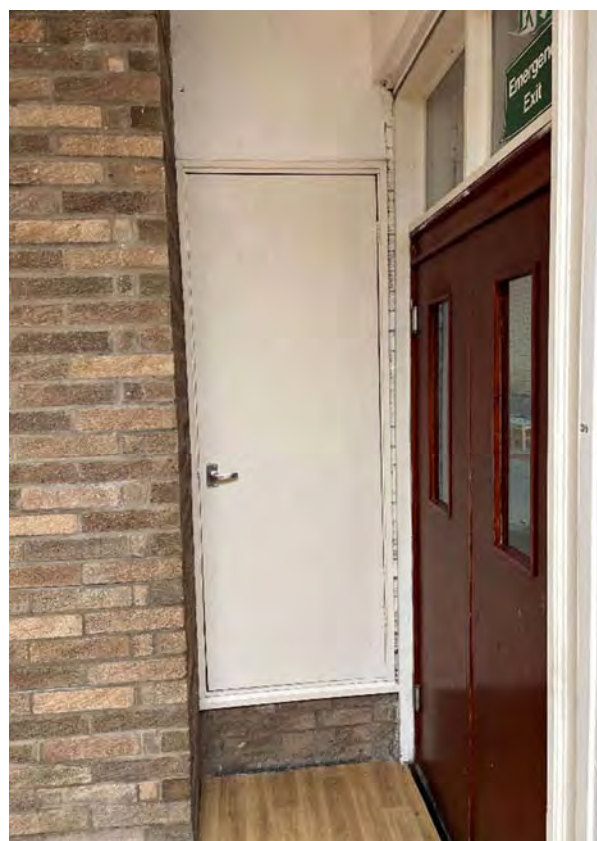
Inadequate clearance in front of fire escape doors.
