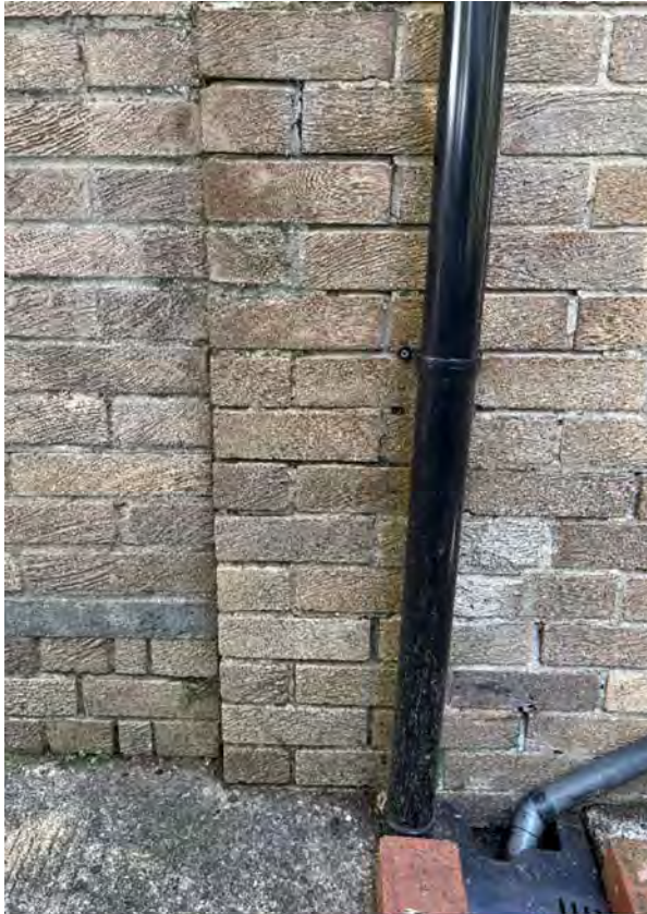
Example area of loss of pointing around downpipe.
