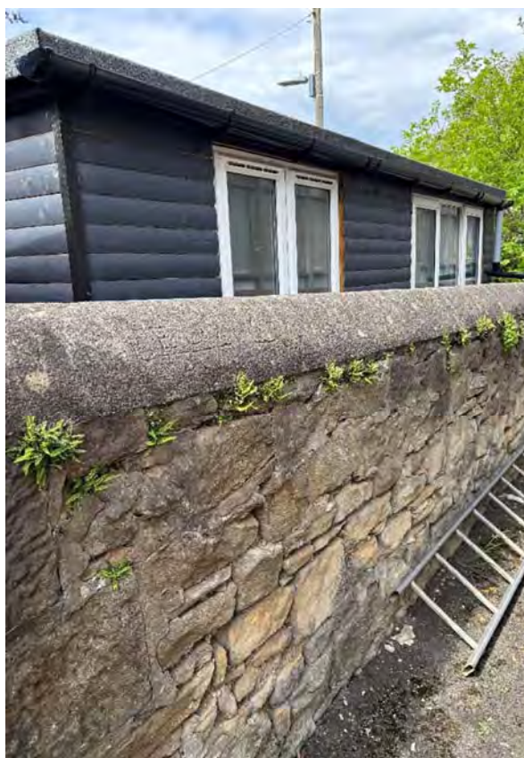
Deterioration of stone boundary wall.
