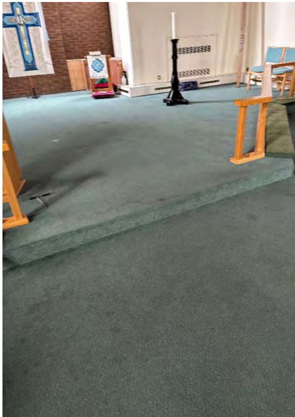
Step up should be identified more clearly to prevent trips.
