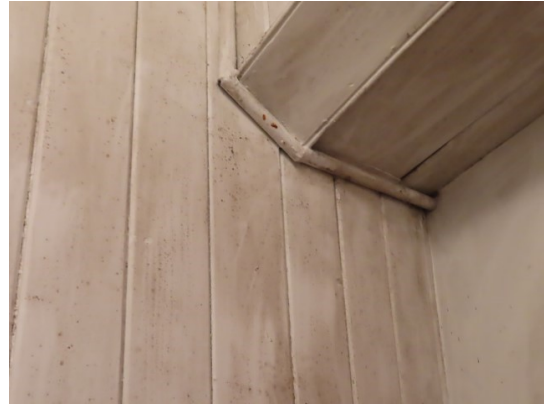
Mildew growth to the timber
