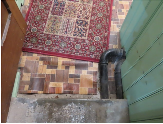
Poorly defined step and projecting pipework to Choir Vestry
