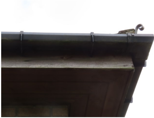
Failing stain finish to Parish room fascia and overhanging eaves
