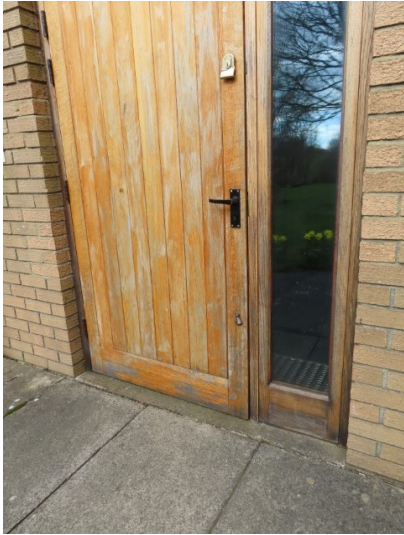
Failing finish to parish room door
