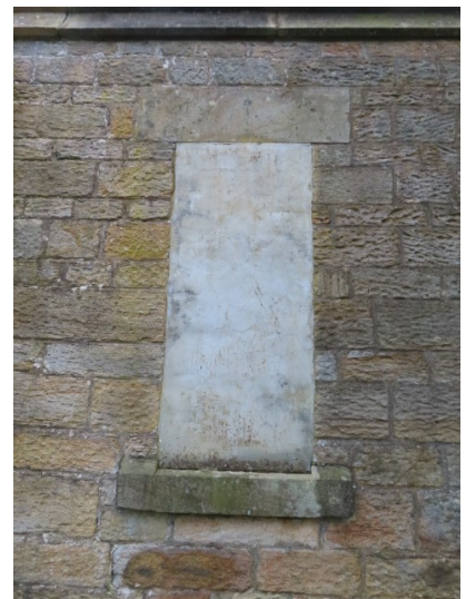
Failing ply finish to Organ Chamber window openings
