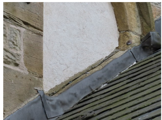
Failed pointing over flashings over link roof
