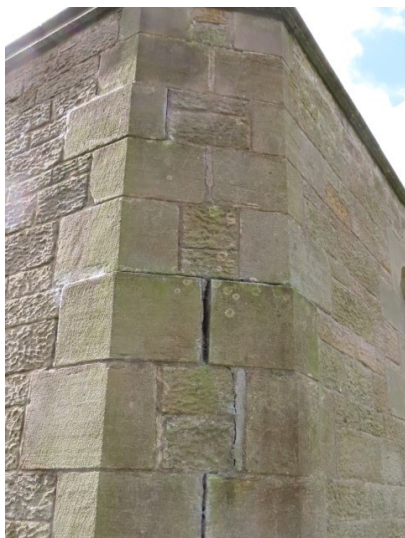
Cracking to North East corner of the Vicars vestry
