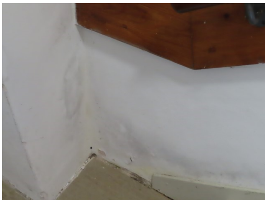
Dampness and deterioration to plaster by steps Parish room
