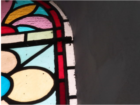
Saddlebar to Sii not fixed into the wall
