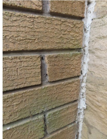
Failing mastic to junction between Parish room/link and the Nave
