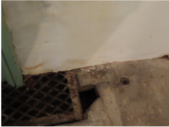
Damaged flag to the side of the grating near the porch
