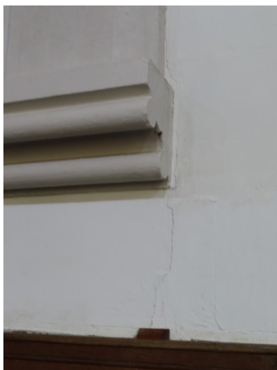
Crack to Chancel wall
