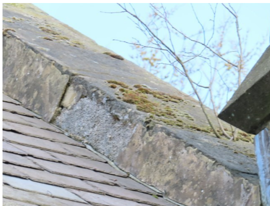
Sapling and failing mortar fillet to the Chancel
