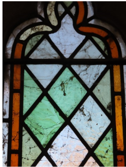
Debris behind window visible internally
