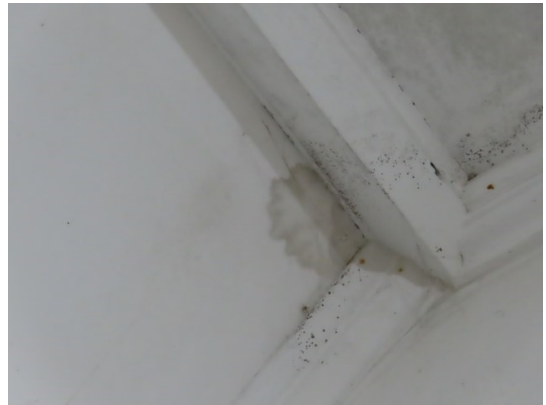
Damp patch to East Chancel ceiling To Chancel
