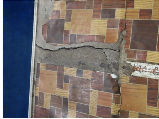
Significant cracking to Choir Vestry floor
