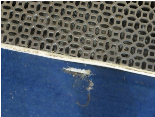
Damage to carpet (possibly due to defect below)
