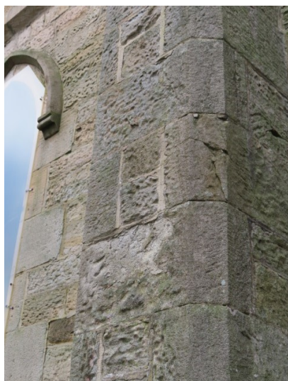
Cracked stone to South East corner of the Nave
