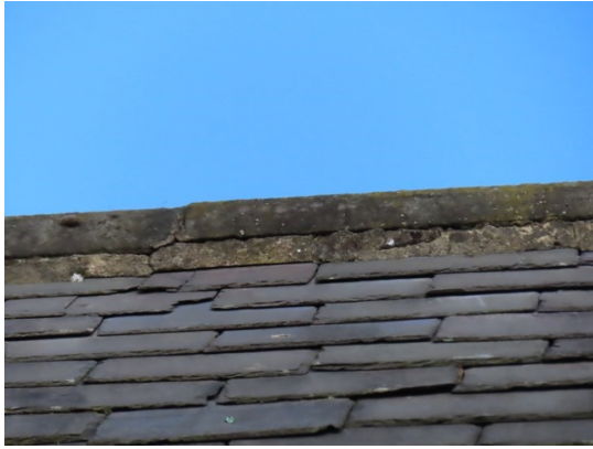
Failing mortar bed to the Chancel roof
