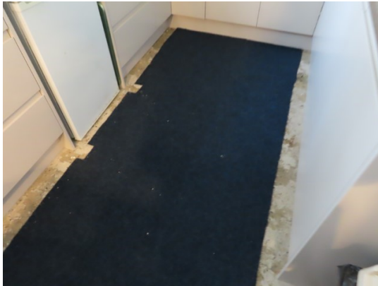
Floor covering in the kitchen is undersized
