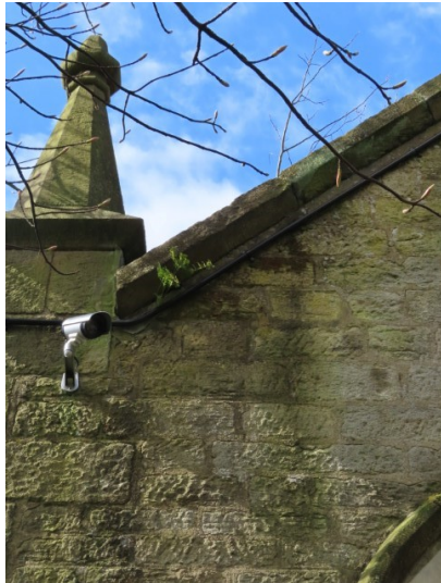
Vegetation & open joints to water table & Pinnacle to East Elevation of the Chancel
