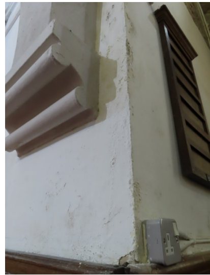
Blistering of paint/plaster to junction between the Nave and Chancel
