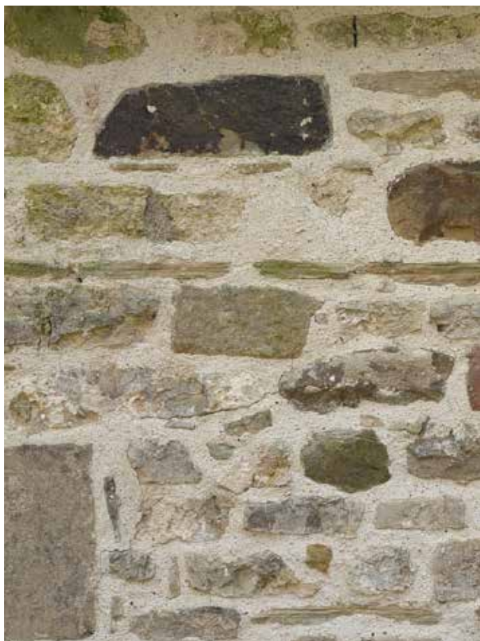
External crack to Thornley Porch
