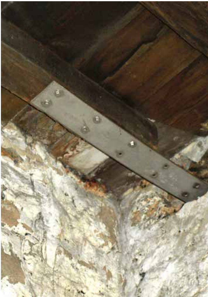
Strap repairs to the embedded timbers are structurally poor and should be re-worked to a Structural Engineer's design
