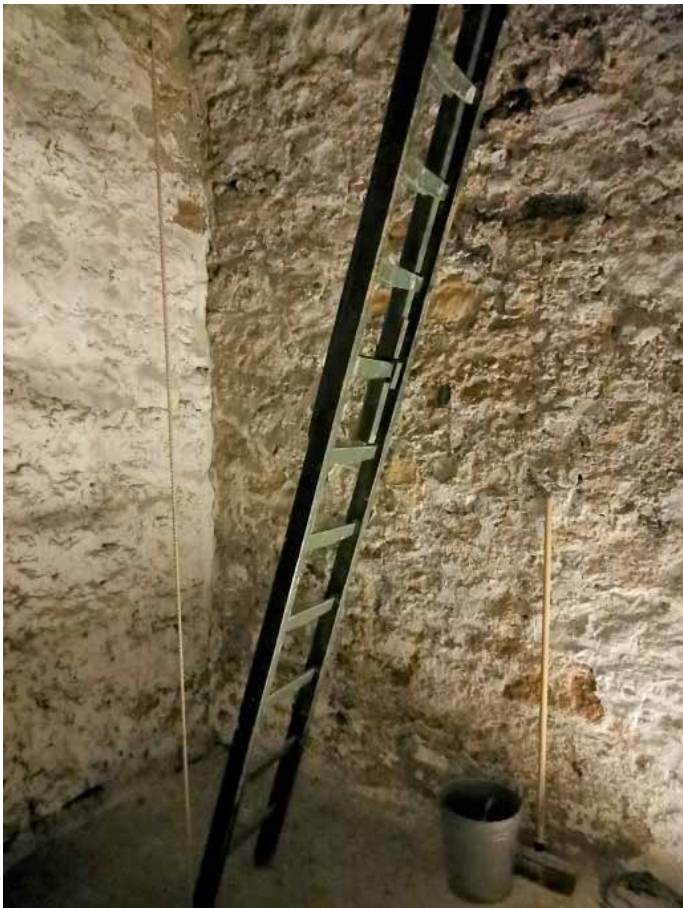
Historic timber ladder should be replaced with alloy or galvanised steel equivalent
