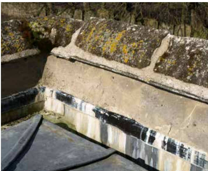
Frost-damaged render to the inside face of the tower parapet
