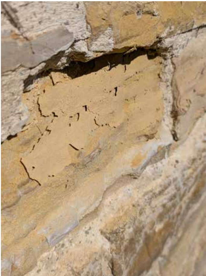
Stone decay is widespread across the building, exacerbated by over-hard pointing in many places.
