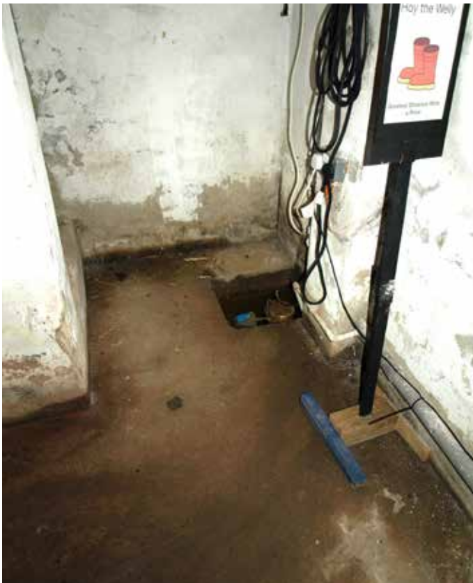
The boiler-room is particularly wet, and roof and abutment details should be checked
