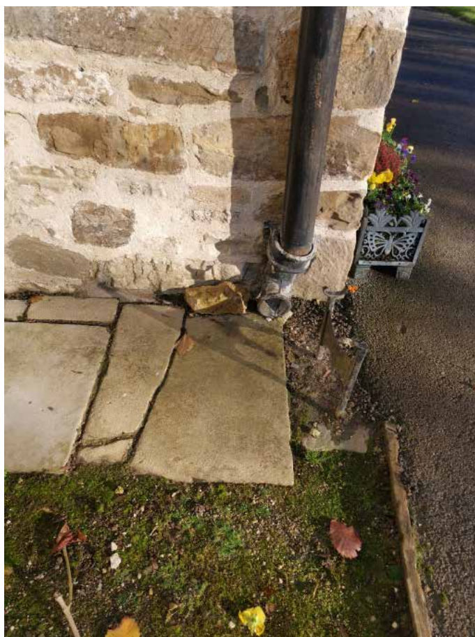
Porch downpipes discharge over ground
