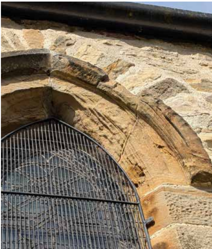
Hoodmould cracking has led to loss of section - the adjacent section is also at risk of failing
