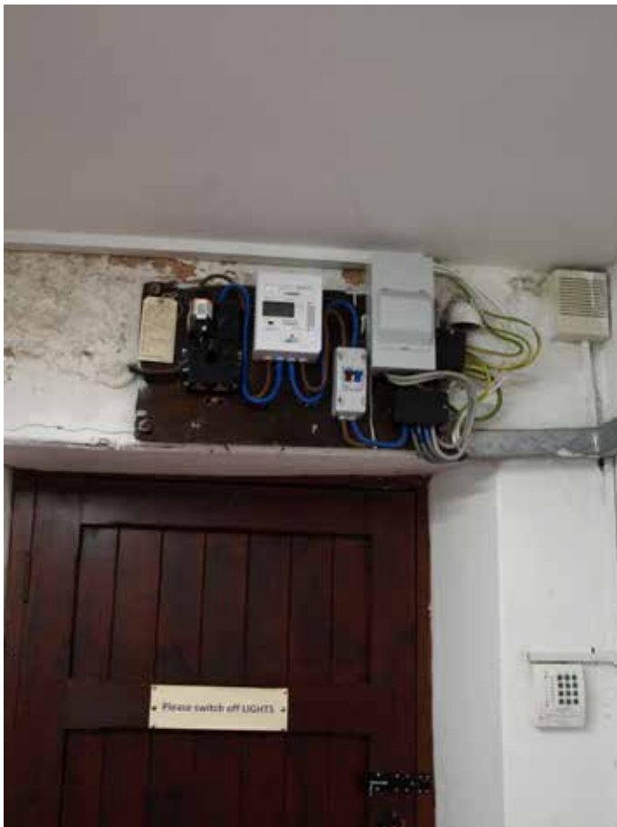
Damp around electrical installation, possibly due to leaks from verge coping stones above.
