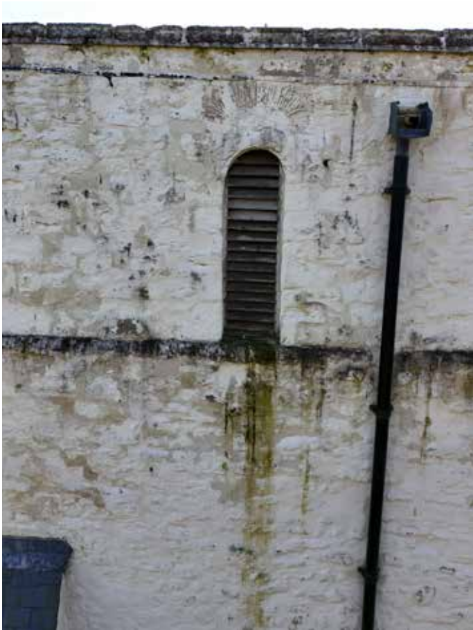
Wear and algae staining to tower limewash
