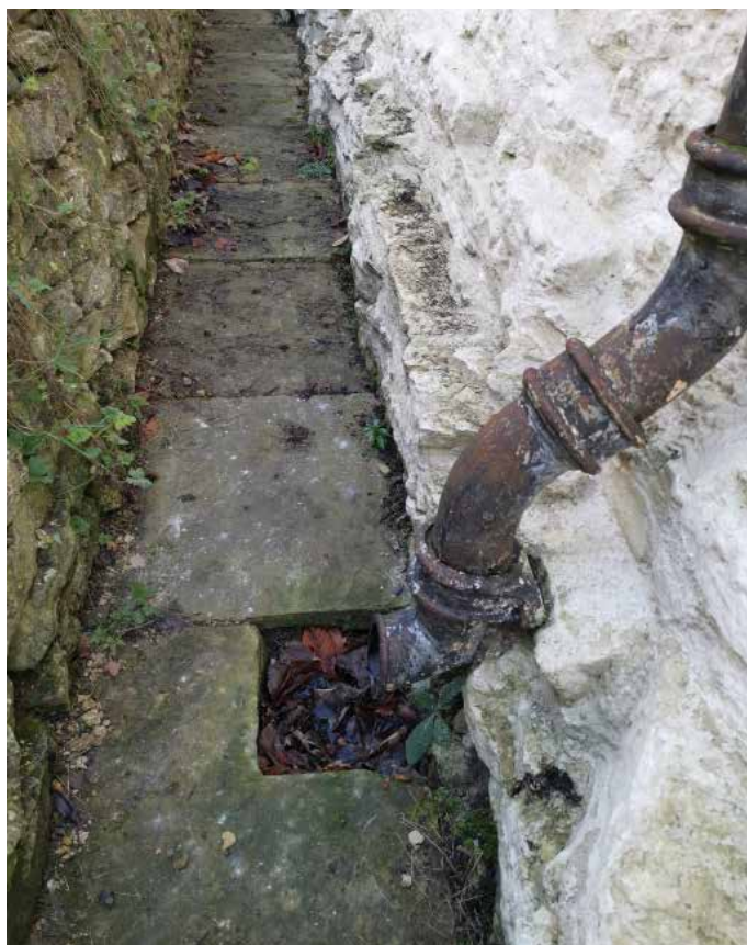
Gullies restricted by leaves, downpipe rusting
