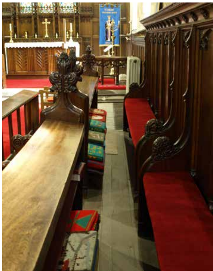
Choir pews on timber platforms - distortion of floor should be investigated.
