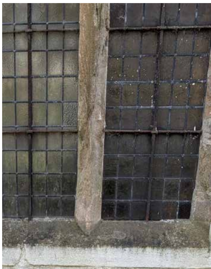
Rusting ferramenta to window
