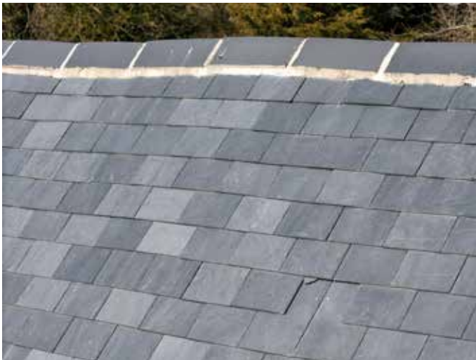
Nave south slope: missing slate, ridge pointing poor
