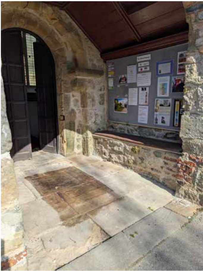
Lifting the rubber-backed matting in the Porch reveals trapped moisture - seen here as a dark damp patch
