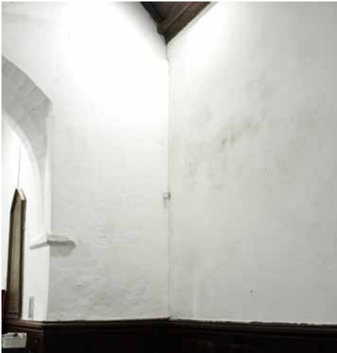
Damp staining and minor mould to nave north wall, to be monitored
