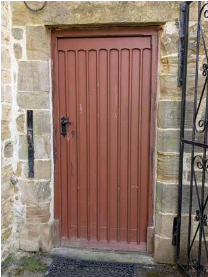
All external doors would benefit from re-painting
