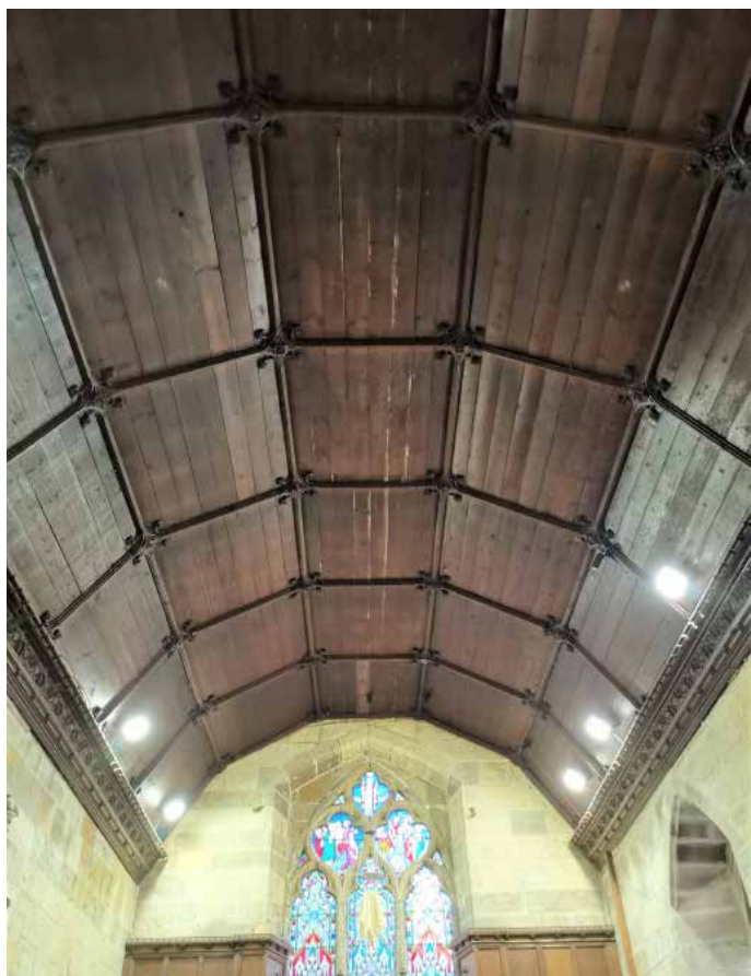
Chancel ceiling, water staining historic
