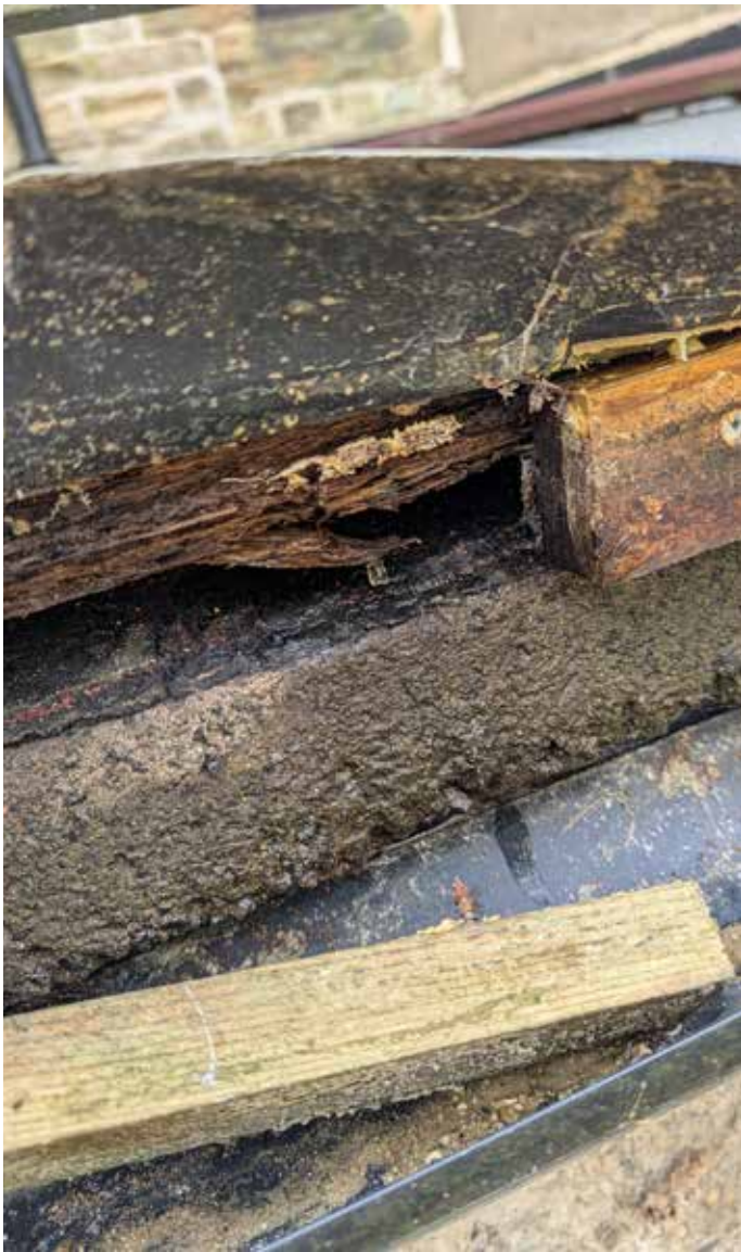
Decay to timber detail of boiler-room roof
