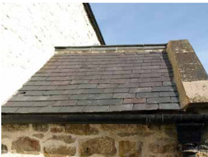
Porch roof, west slope: broken, damaged & displaced slates
