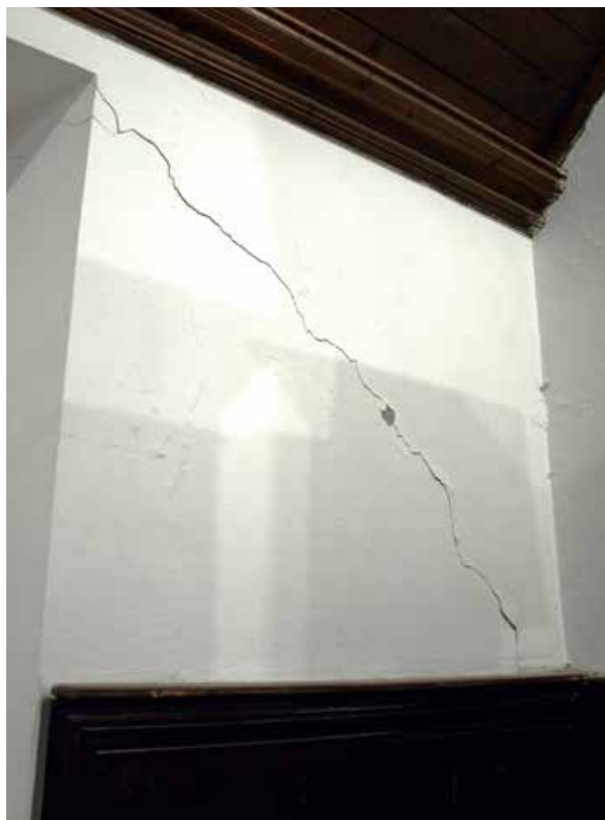
Cracking in the Thornley Chapel should be investigated
