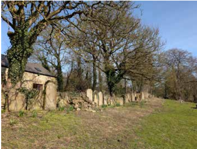
Headstones fixed along the north boundary wall. Area of collapsed wall
