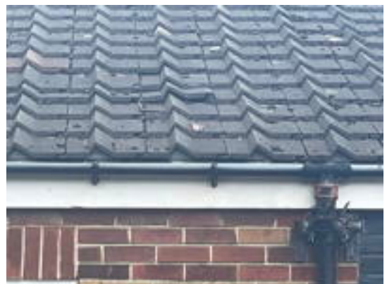
Displaced Tile to Hall Roof East Elevation
