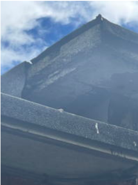
Choir Vestry/ Meeting Room Spalling Concrete at South West Corner
