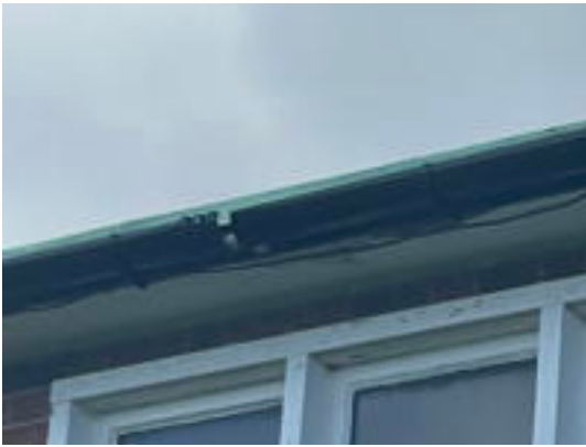
Open Joint to Gutter North
