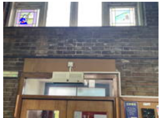
Salts above North Porch
