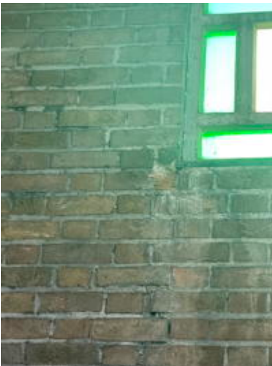
Open joints and Staining to West Window
