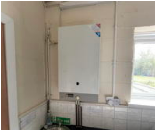
Hall Kitchen Water Heater
