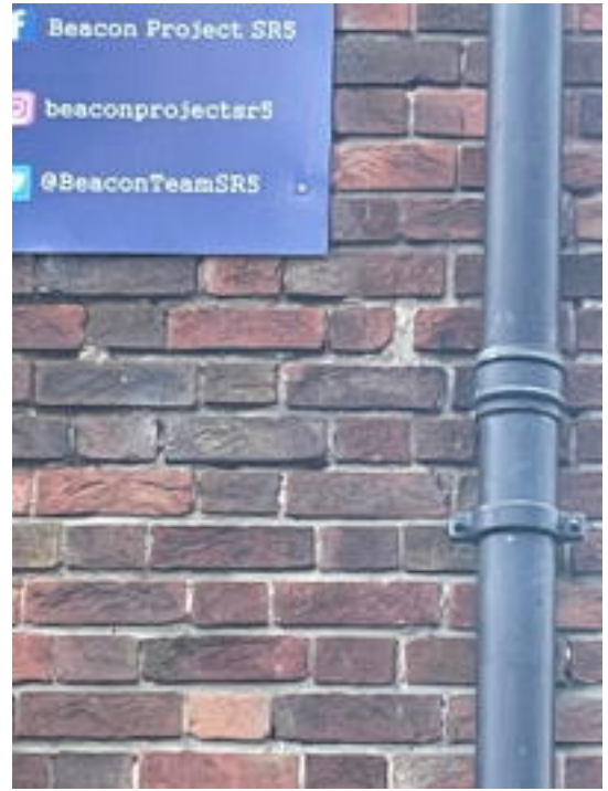
North Elevation Inadequate Pointing
