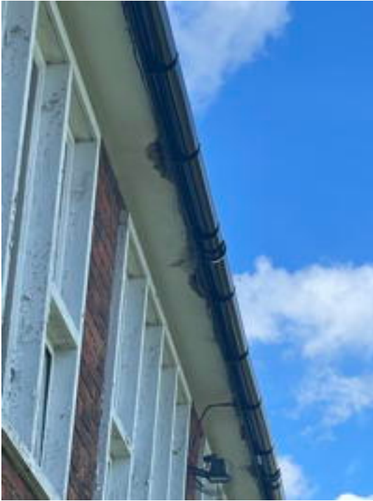
North Elevation Spalling Concrete at Eaves
