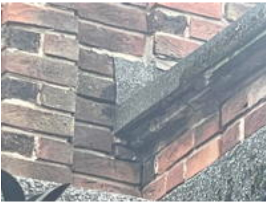
Choir Vestry/ Meeting Room Spalling Concrete West Elevation
