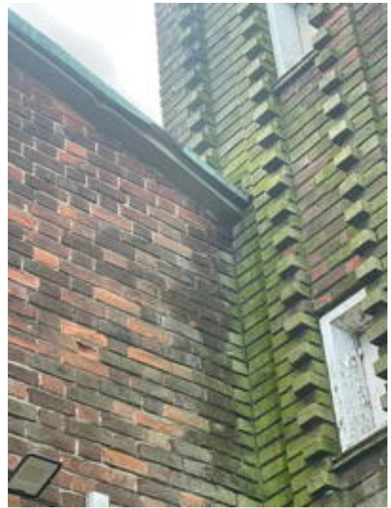
West Elevation Spalling Concrete at Eaves
