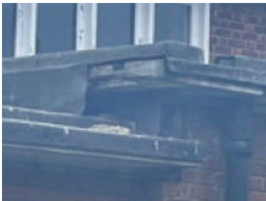
Missing Felt and Spalled Concrete to Choir Vestry/Meeting Room Roof
