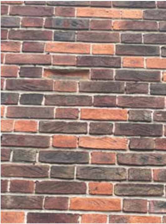
West Elevation Spalled Brickwork
