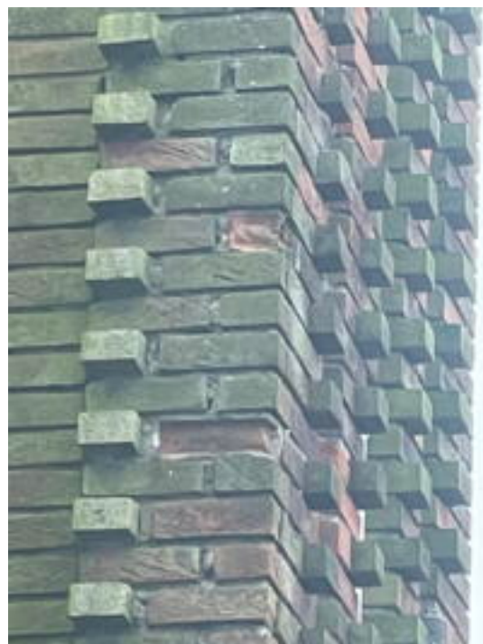
Tower North West Corner Spalled Brickwork
