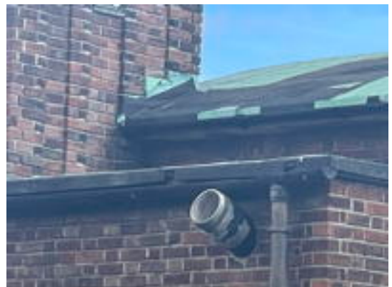
Missing Felt to Organ Loft Roof
