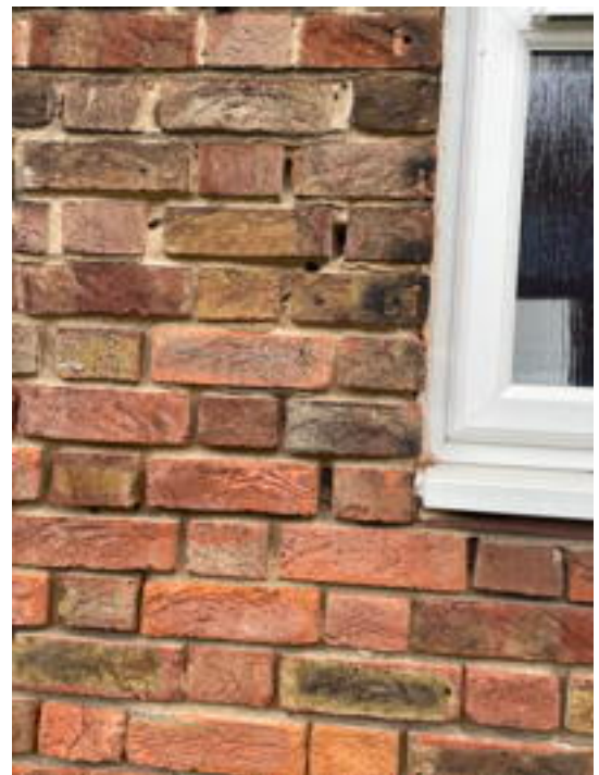
Meeting Room/Choir Vestry South Elevation Inadequate Pointing
