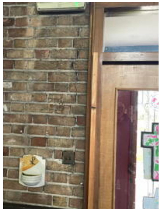
Cracking at North Porch Doors Left Hand Side
