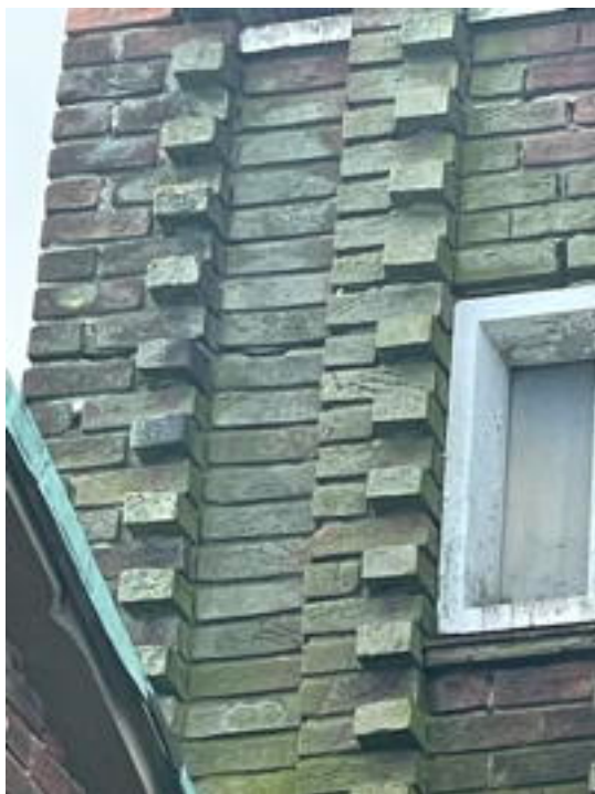
Tower North Elevation Horizontal Cracking
