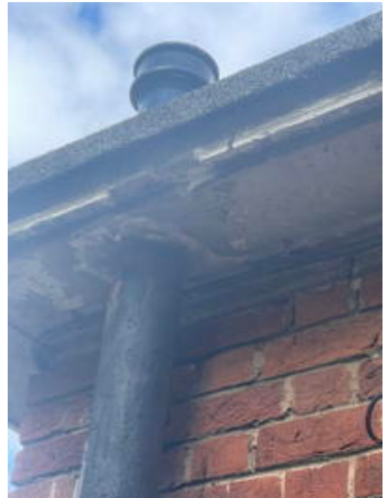
Choir Vestry/ Meeting Room Spalling Concrete South Elevation
