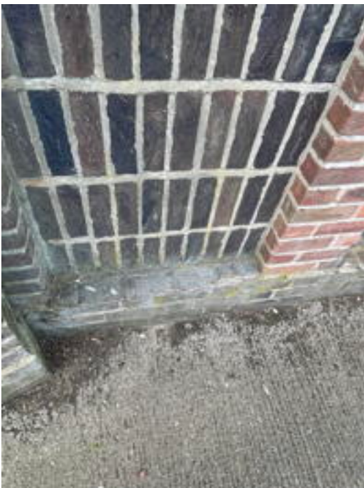
Broken Creasing Tiles to Base of Sanctuary Brickwork
