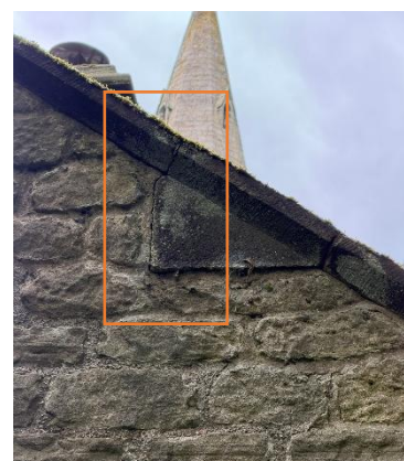
Figure 11 – East Vestry cracking
