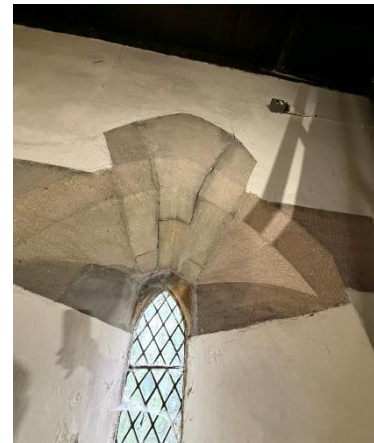
Figure 22 - crack at head of west window
