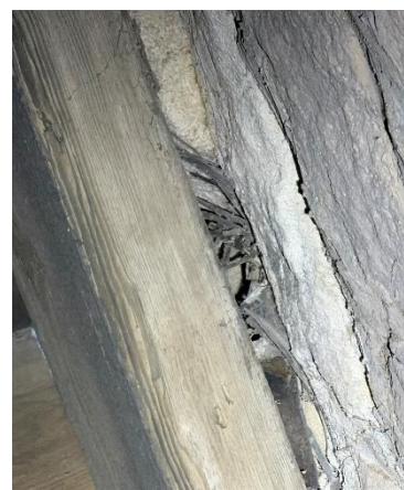
Figure 18 - gap in belfry ceiling boarding
