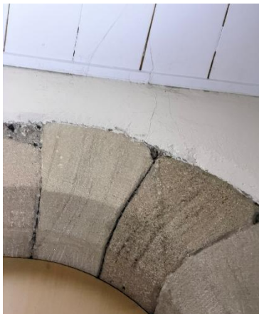
Figure 20 - crack to circular window
