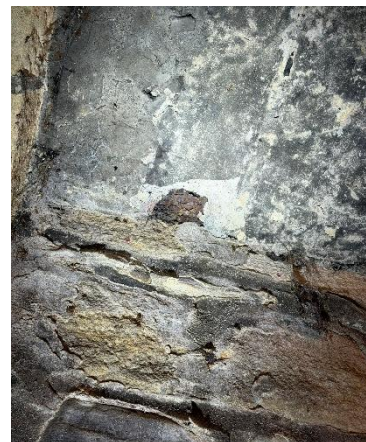
Figure 17 - Rust to ceiling
