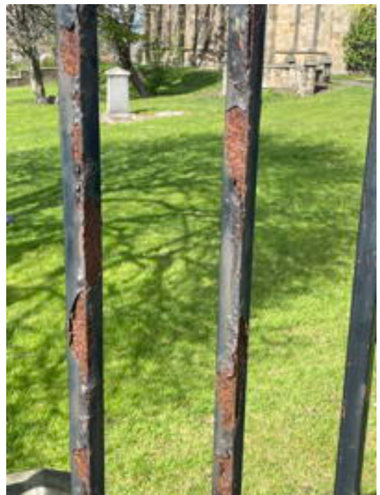
East Elevation Typical Rusting Railings
