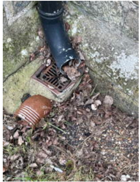
Gully Not Connected to Drain
