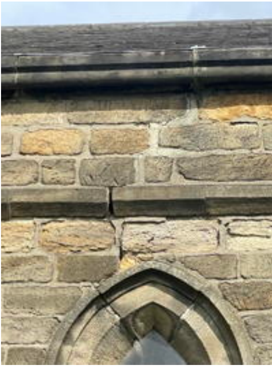
Chancel South Elevation Open Joints and Eroding Stonework
