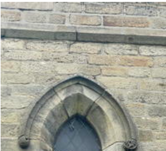
North Elevation Cracking
