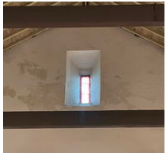
Nave East Residual Damp
