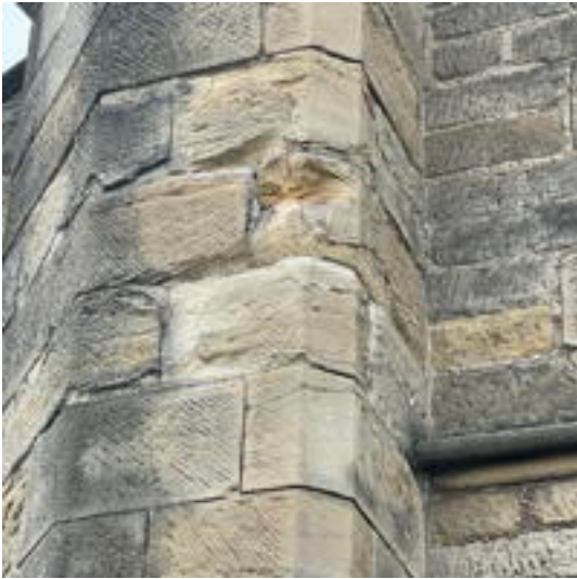
Tower West Elevation Eroding Stonework to Buttress
