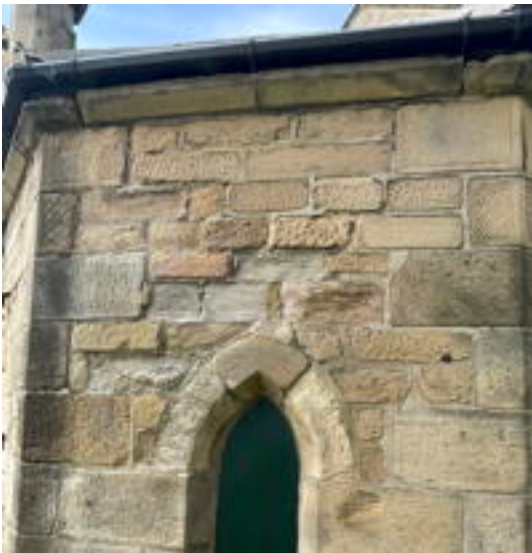
Vestry North East Elevation Eroding Stonework
