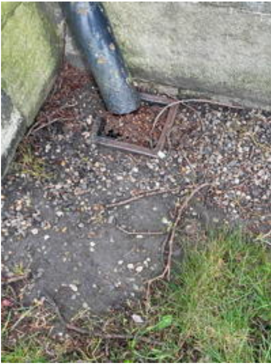
Gully Partially Blocked by Leaves
