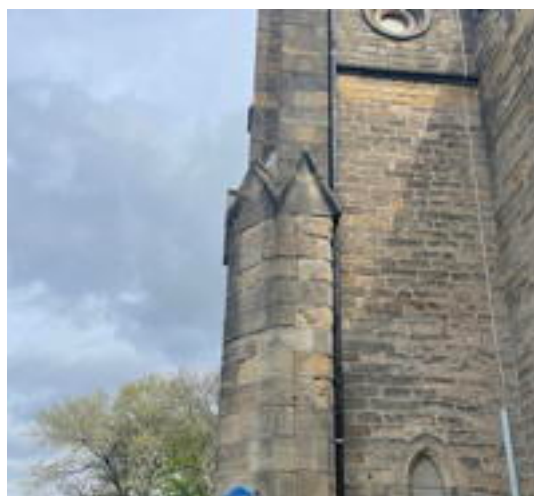
Tower South Elevation Eroding Stonework to Buttress
