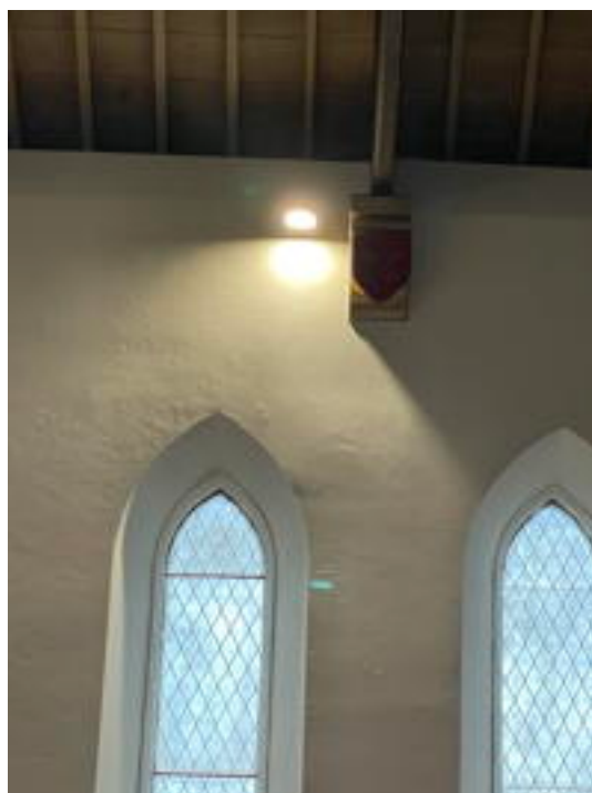
Typical Nave Light
