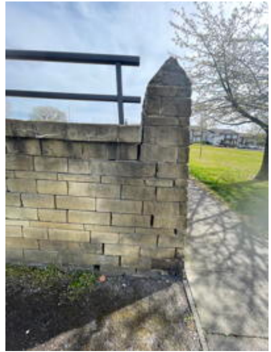
South West Corner Movement
