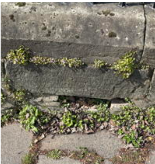
East Elevation Wall Typical Missing Pointing Plant Growth
