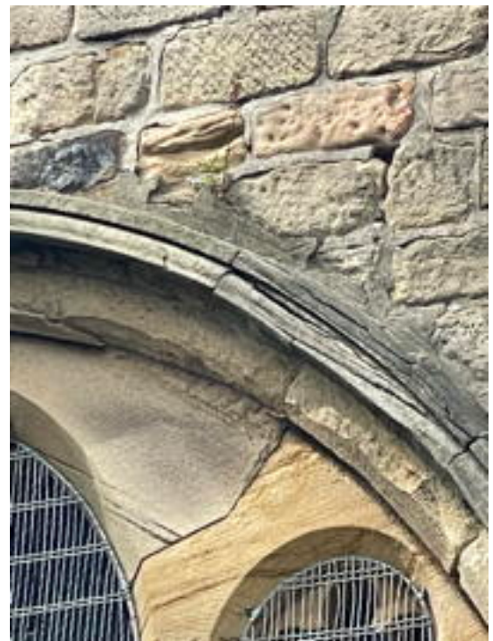
Chancel East Elevation Open Joints and Eroding Stonework
