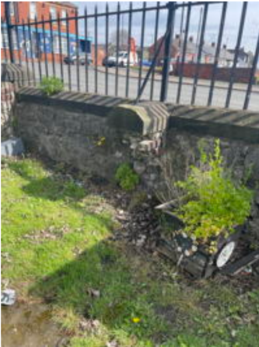
Collapsed Buttress East Elevation
