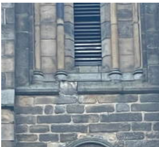
Tower West Elevation Fallen Stone
