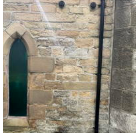
Vestry North Elevation Eroding Stonework
