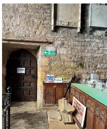
Figure 56 - Algae build up at N Door
