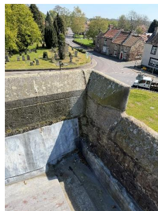
Figure 1 - loose parapet SE
