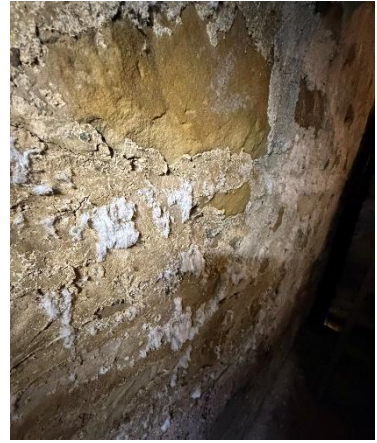
Figure 41 - salts on wall
