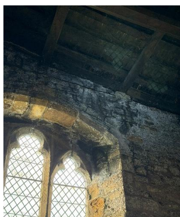
Figure 55 - W window with leak
