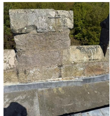
Figure 10 – Lead flashing failure
