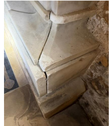
Figure 62 - opening joint to monument
