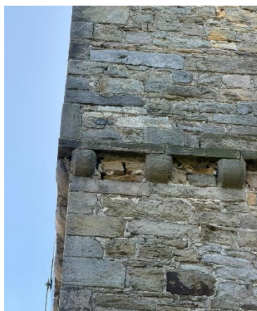
Figure 33 - N erosion at corbel
