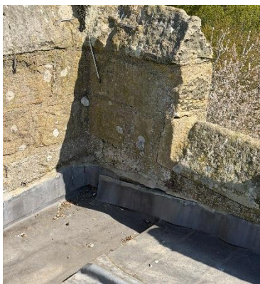
Figure 11 – lead flashing failure
