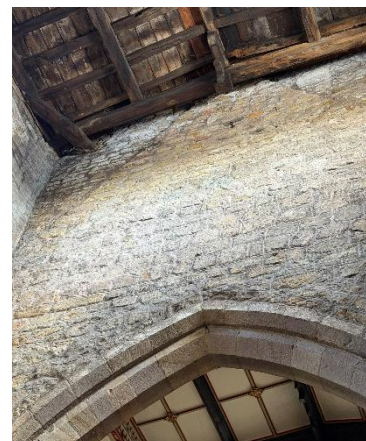
Figure 54 - High level efflorescence
