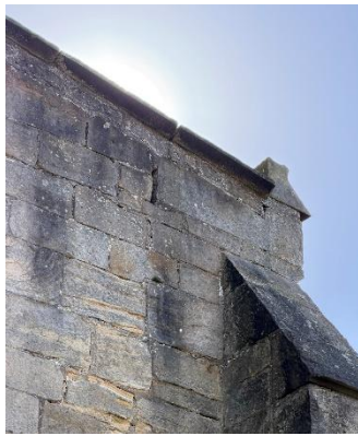
Figure 26 - W end S Aisle open joint
