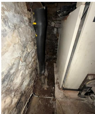
Figure 46 - Erosion to W wall boiler
