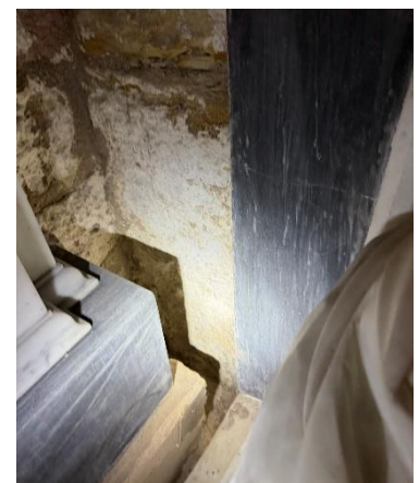
Figure 63 - Damp in NW corner
