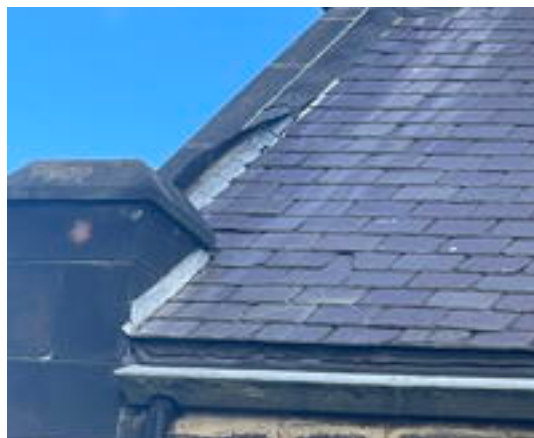
Loose Parapet Flashing Nave West End South Elevation
