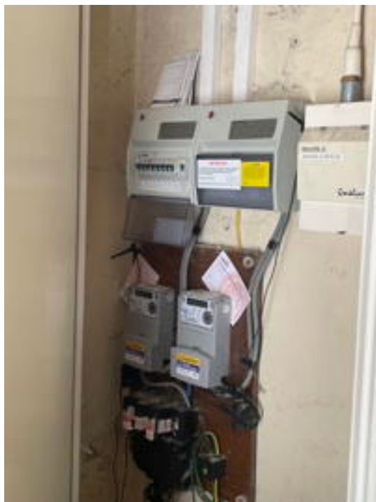
Entrance Porch Meters and DB Boards
