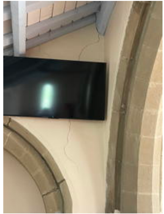
Cracking North Aisle East End
