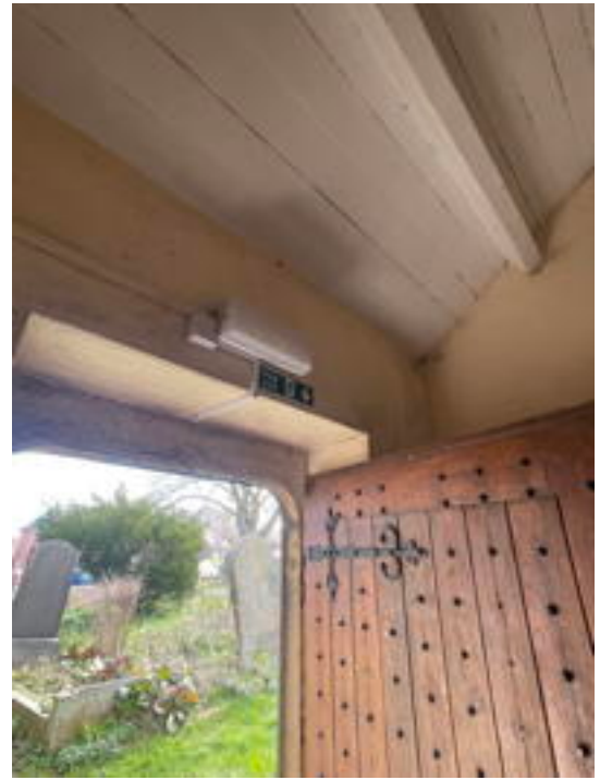
Deteriorating Paintwork Door Head
