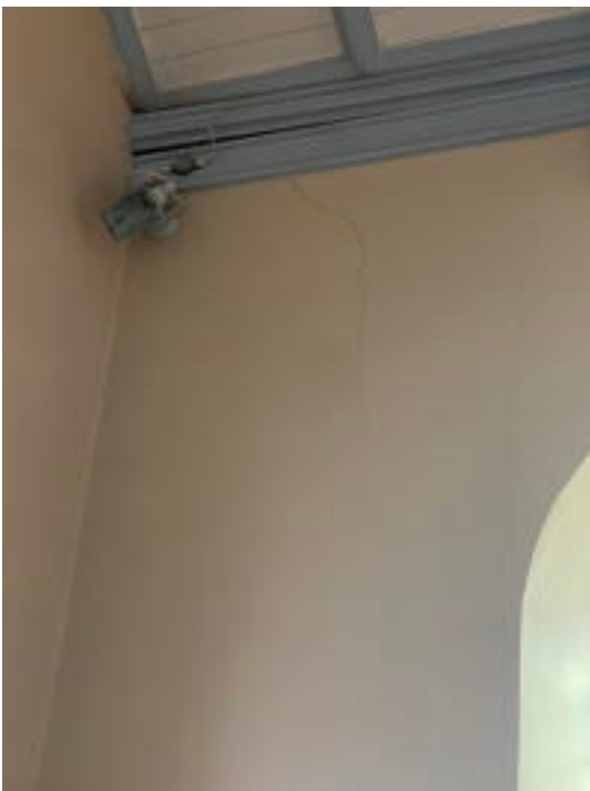
Cracking at Eaves
