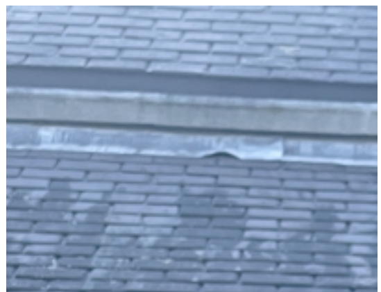
Lifted Flashings North Roof
