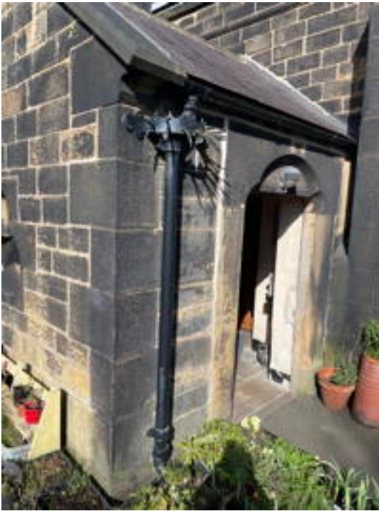
Porch Rainwater Pipe
