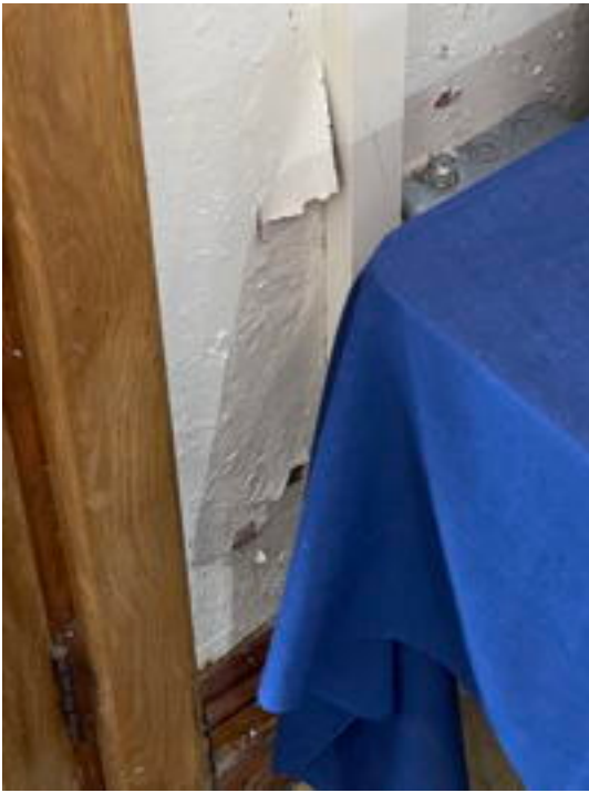
Peeling Paint at Porch Door
