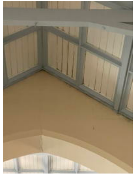
Minor Staining to Chancel Roof
