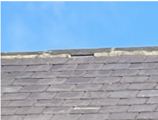
Chancel South Roof Missing
