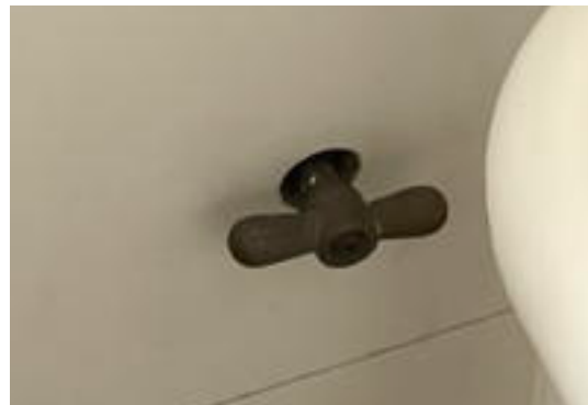
Assumed Incoming Water Mains Isolation Tap in WC
