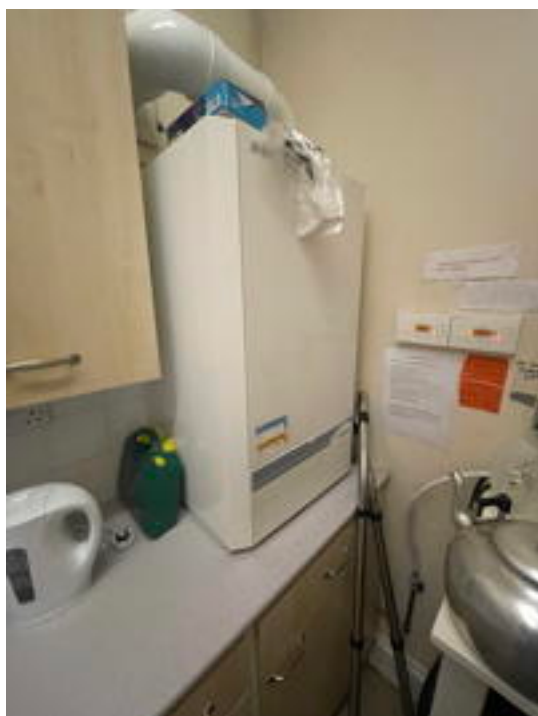
Boiler in Kitchen
