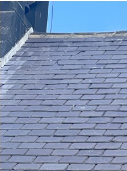
Broken Slates South Nave Roof
